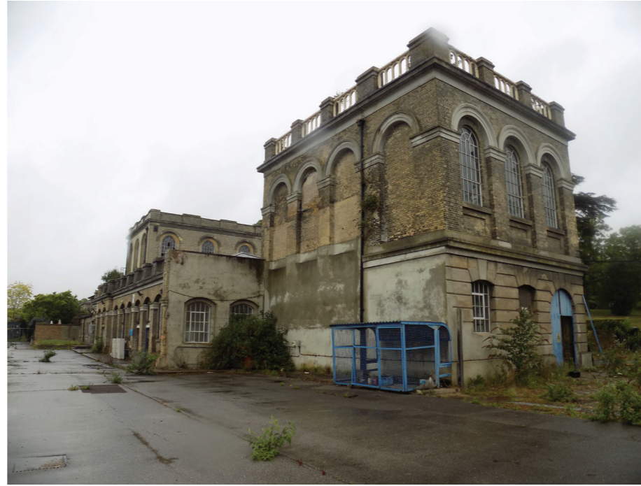
Figure 133: Karslake East Bull Engine House showing cement repairs where former warehouse building has been removed.
