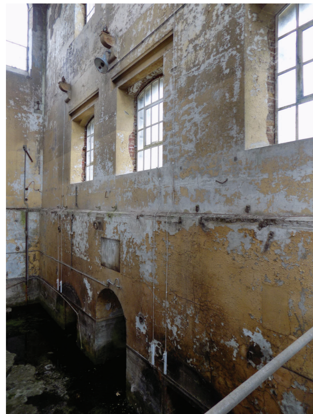
Figure 136: Interior detail showing below ground level and later inserted windows at ground floor level.
