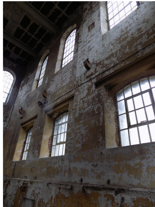
Figure 137: Interior showing original windows at upper level and 1930s windows at ground floor level.
