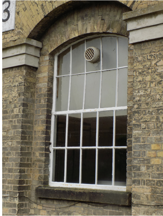
Figure 132: Karslake Boiler House, South Elevation. Cast Iron window, showing slight bow indicating a high degree of repair might be required.
