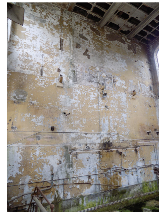
Figure 141: Interior detail showing fittings for Bull Engine installation.
