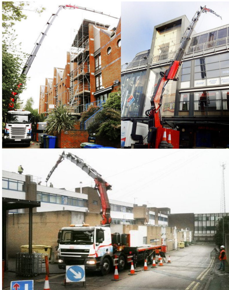
Images of typical hiab crane lifting and distribution materials onto an existing roof
