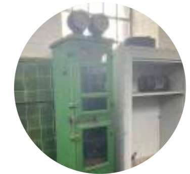
Item 8 Harland control cabinet for electric centrifugal pump Low to medium significance
