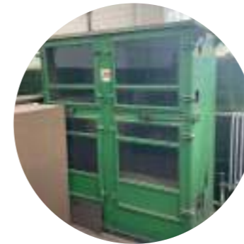
Item 6 Harland control cabinet for electric centrifugal pump Low to medium significance
