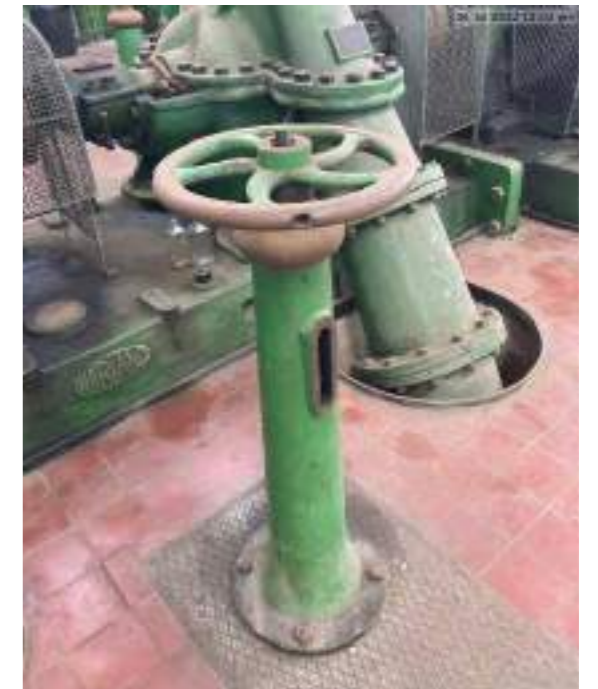
Valve Control standard for centrifugal pump Date: 1932 Size: 0.4 d Report comment: Low to medium significance
