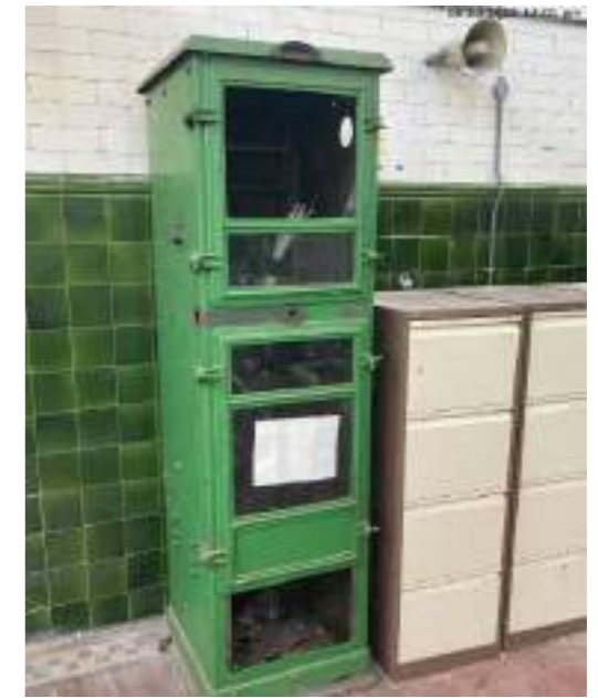
Harland control cabinet for electric centrifugal pump Date: 1932 Size: 0.6m x 0.6m Single Leaf Report comment: Low to medium significance
