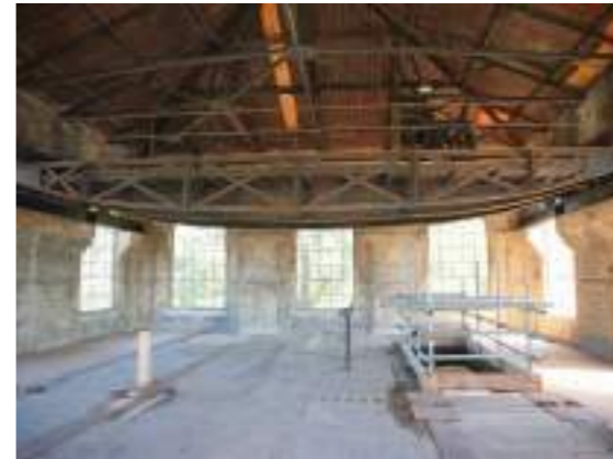
Top level 3 of the western block, 'The Beam,' with a large steel gantry crane and steel trusses
