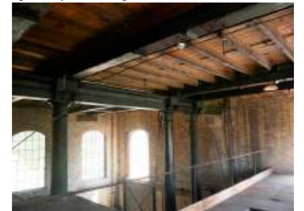
Tuscan order steel columns hold up the second floor's large steel beams in The Beam
