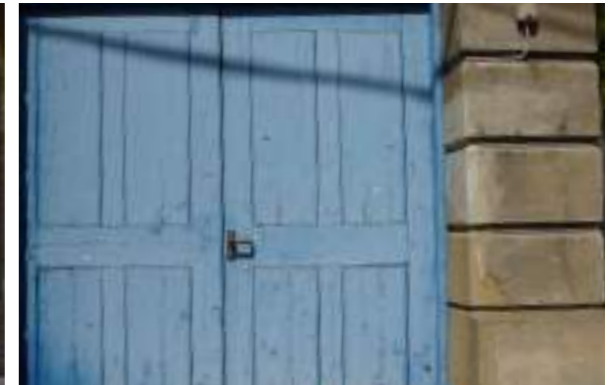
The royal blue timber doors add highlight the entrances and provide a contrast with the stonework
