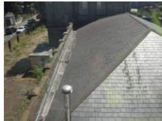
View from the western block, looking over the slate roof of the central single storey block
