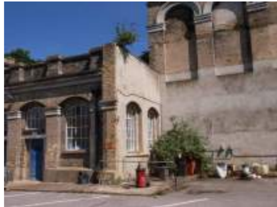
An area at the SE corner of the building, where a previous extension has since been demolished in 1977
