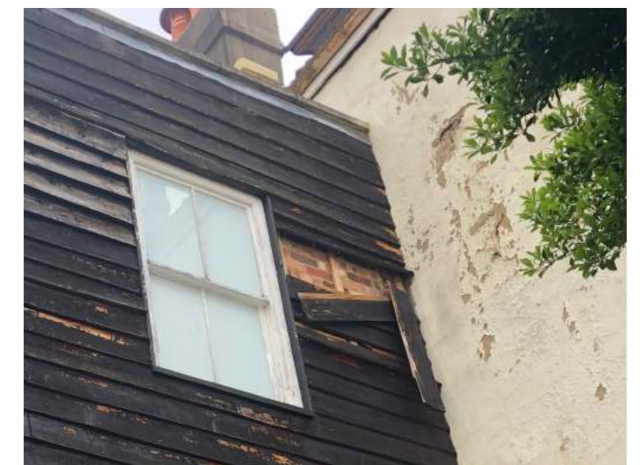
Damaged timber cladding to be removed
