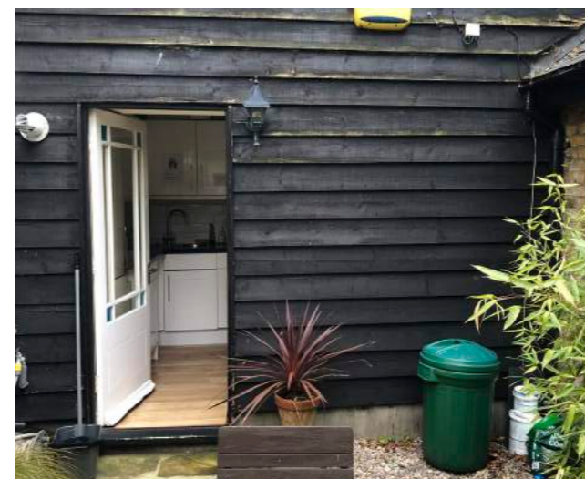
Existing door to be replaced with glazing
