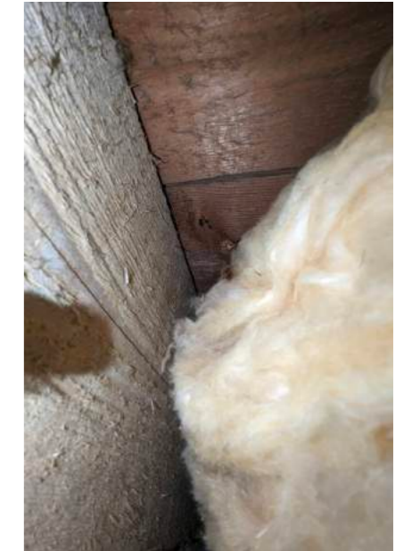
Flat Roof Construction - view through light fitting aperture. Square edged joists overlaid with timber boards.
