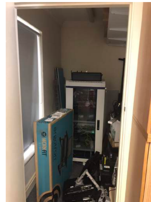
Existing server room
