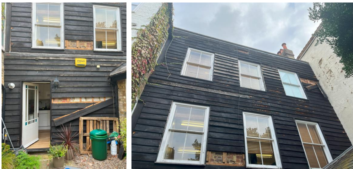
Figures 6 and 7: Views of the rear elevation of 31 The Green with some areas of opening up
