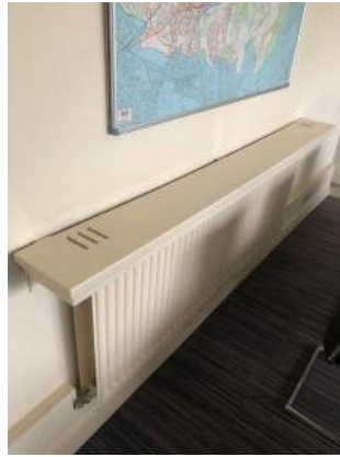
Existing radiator and shelving
