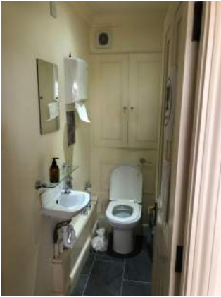
Existing WC sanitaryware
