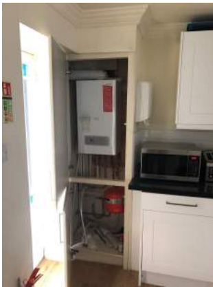
Existing boiler location
