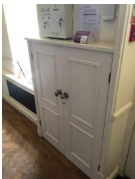
Existing electrical cupboard
