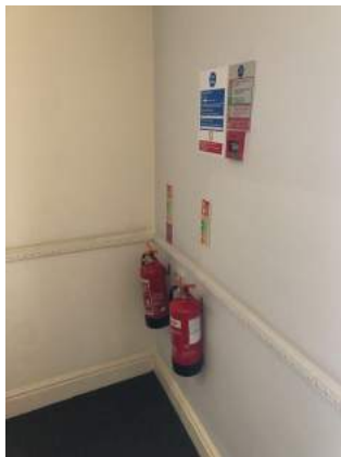
Existing Fire extinguisher points
