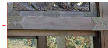
Areas of damage to lacquer, repair and refinish.
