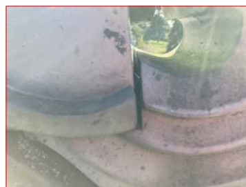
Ridge element slipping slightly
