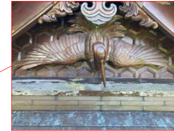
Gable sills subject to weather and could be considered for copper cladding subject to suitable detailing
