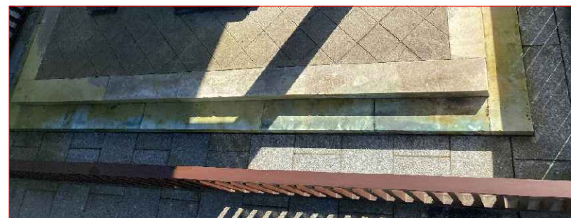
The steps are suffering from copper staining all around the roof perimeter
