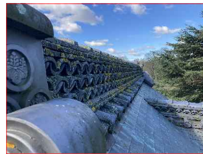
Moss growth to north face of ridge
