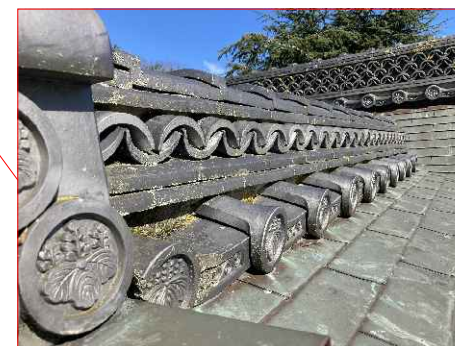
Moss growth to south east of lower ridge
