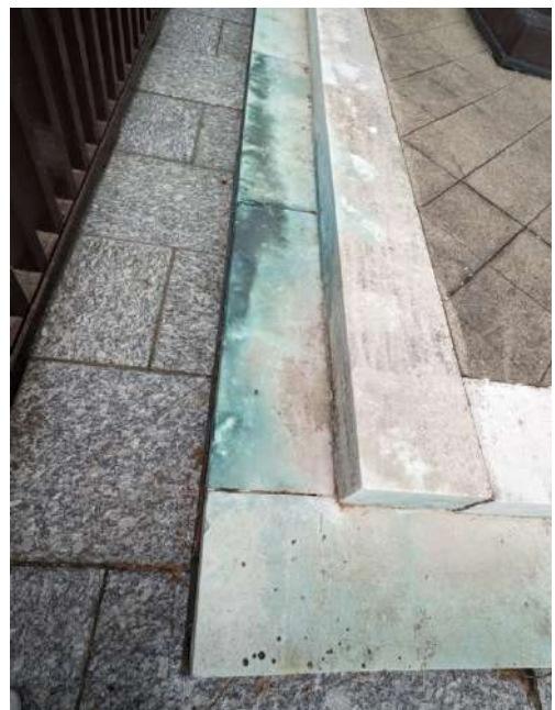
Fig. 11 Copper staining to pavement in south east corner
