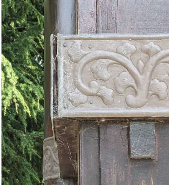
Fig. 8 Split in bracket on the south east corner
