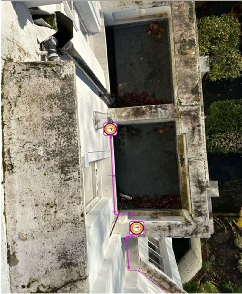
Figure 2: Outlet 2 connection to property, concealed behind existing balcony. Photograph taken from above.
