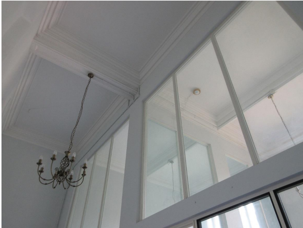
Figure 24: Ground floor – One of the rooms accessed from the north-west corridor. Note ceiling, and modern partitions.
