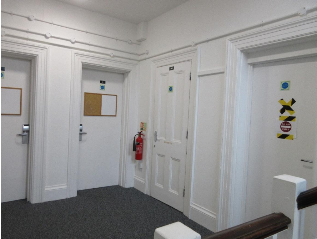
Figure 113: First floor of Red House – Landing. Note original skirting and architraves, and one original door. Note also modern fire doors, and unsightly modern wiring.
