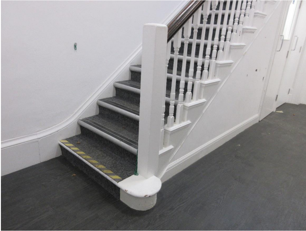
Figure 105: Ground floor of Red House – Stair hall. Note modern treads and risers and skirting to the staircase, and the modern newel post and balustrading. Note also modern skirting to boxing beneath staircase.
