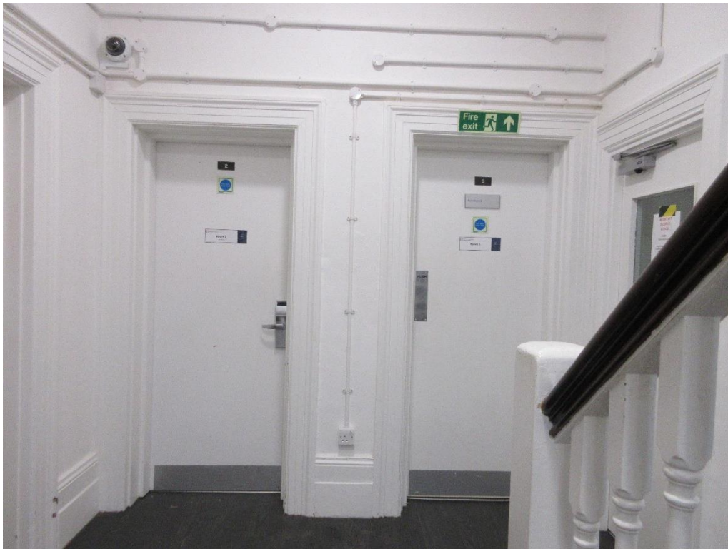
Figure 106: Ground floor of Red House – Stair hall. Note original skirting and architraves, and modern fire doors. Note also the unsightly modern wiring.
