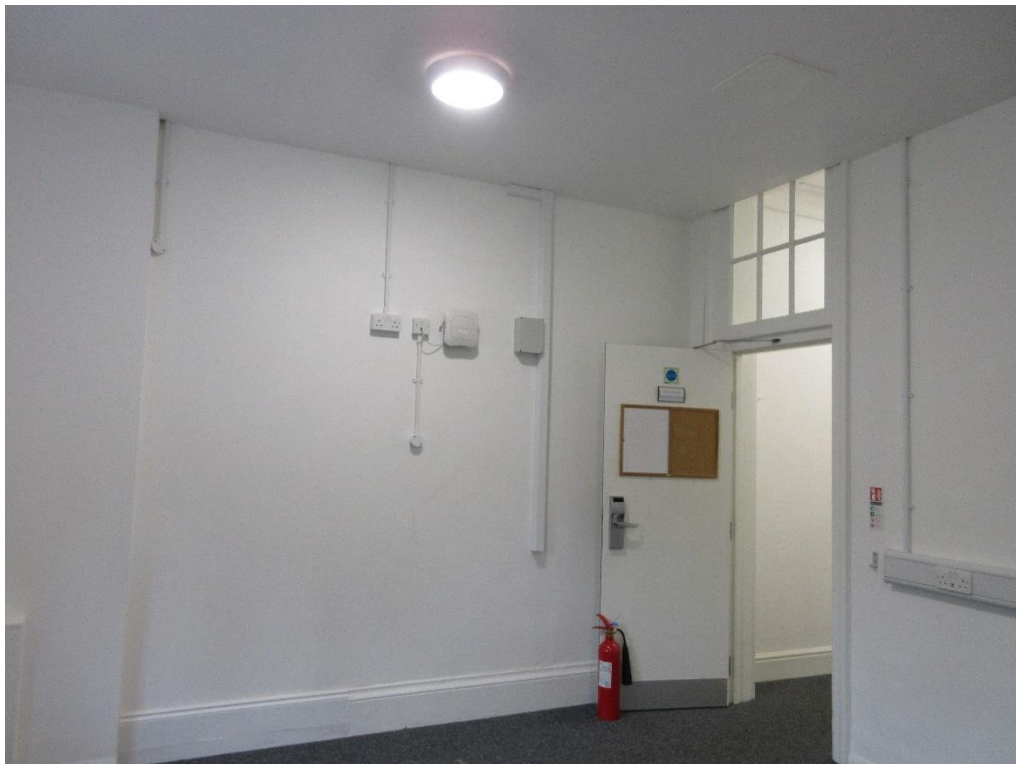
Figure 112: Ground floor of Red House – North-west room. Note modern borrowed light which has been cut off at the top by the modern lowered ceiling. Note original skirting and some replacement modern skirting. Note also the unsightly modern wiring and boxing-in.
