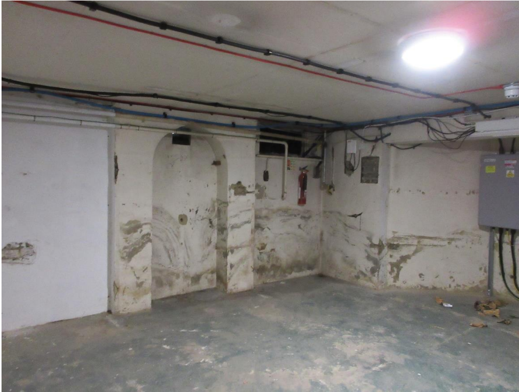
Figure 115: Basement of Red House. Note original chimney breast, and window. Ceiling appears to have been lowered.
