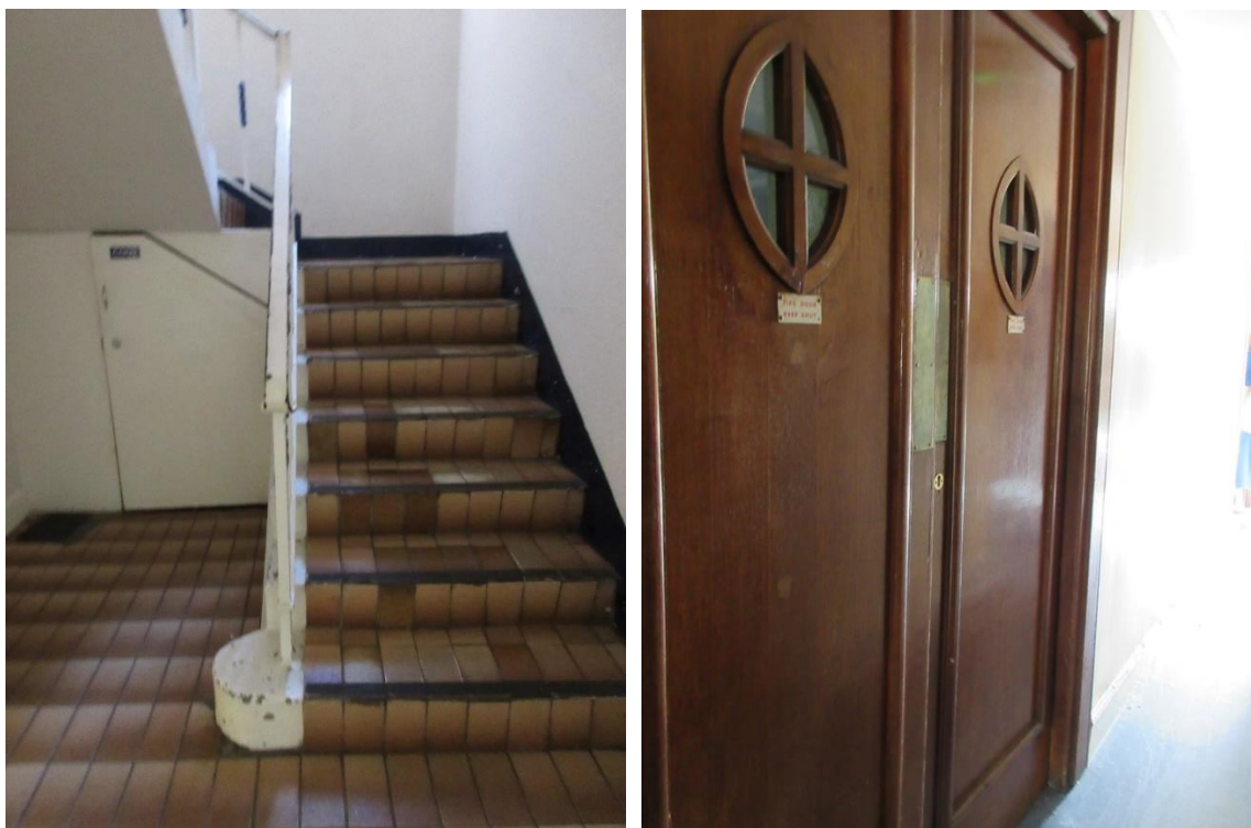
Figure 91 (left): Stairs from basement floor to ground floor in extension B. Figure 92 (right): First floor of extension B.
