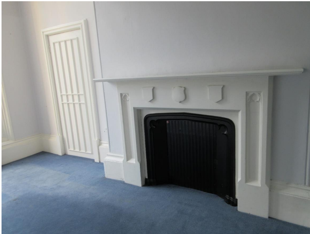
Figure 21: Ground floor – One of the rooms accessed from the north-west corridor. Note original door, chimney breast and fireplace.
