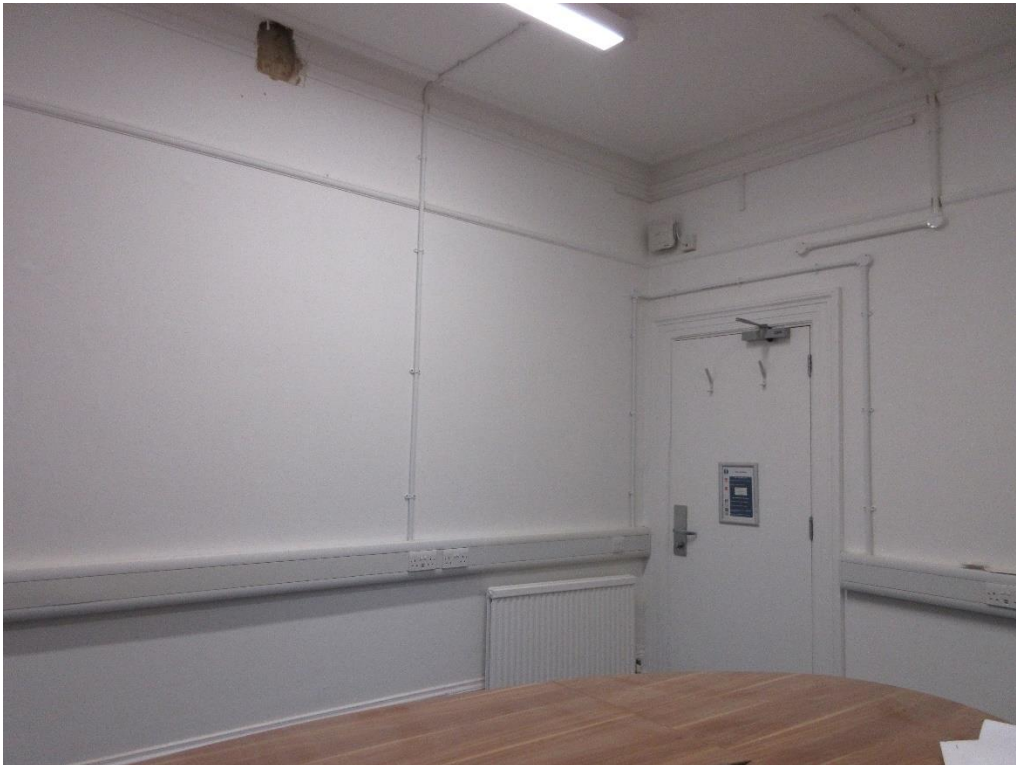
Figure 108: Ground floor of Red House – South-east room. Note original skirting, cornicing and picture railing, door architrave. Note also modern door, and unsightly modern wiring and boxing-in. The proposals involve the provision of a new opening to this wall (between the south-east and south-west rooms).
