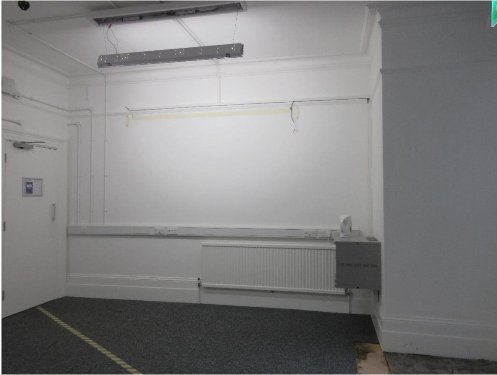
Figure 109: Ground floor of Red House – South-west room. Note original skirting, cornicing and picture railing, and architrave. Note also modern door, and unsightly modern wiring and boxing-in. The proposals involve the provision of a new opening to this wall (between the south-west and south-east rooms).
