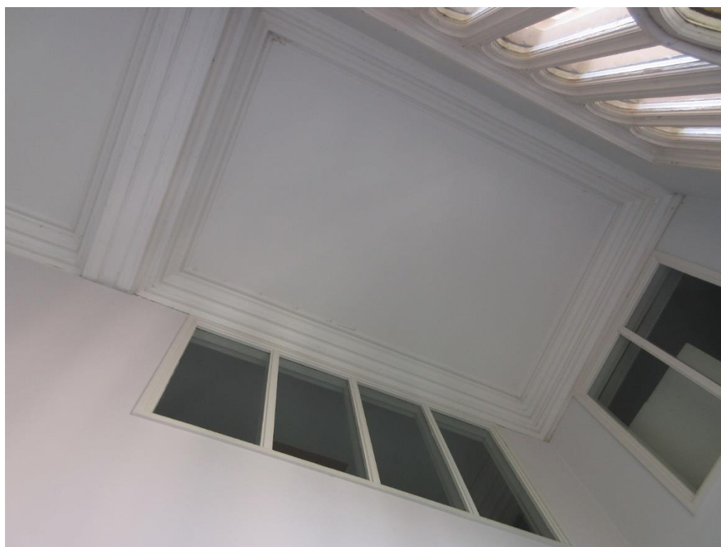
Figure 16: Ground floor – Full-height part of one of the rooms accessed from the north-west corridor.
