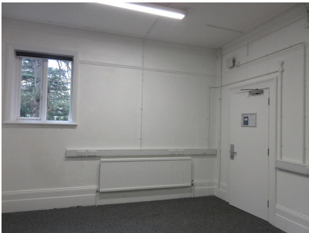
Figure 110: Ground floor of Red House – North-east room. Note original skirting, cornicing and picture railing, and architrave. Note also modern door, and unsightly modern wiring and boxing-in. The windows are likely to be modern replacements. The proposals involve the provision of a new opening to this wall (between the north-west and south-east rooms).
