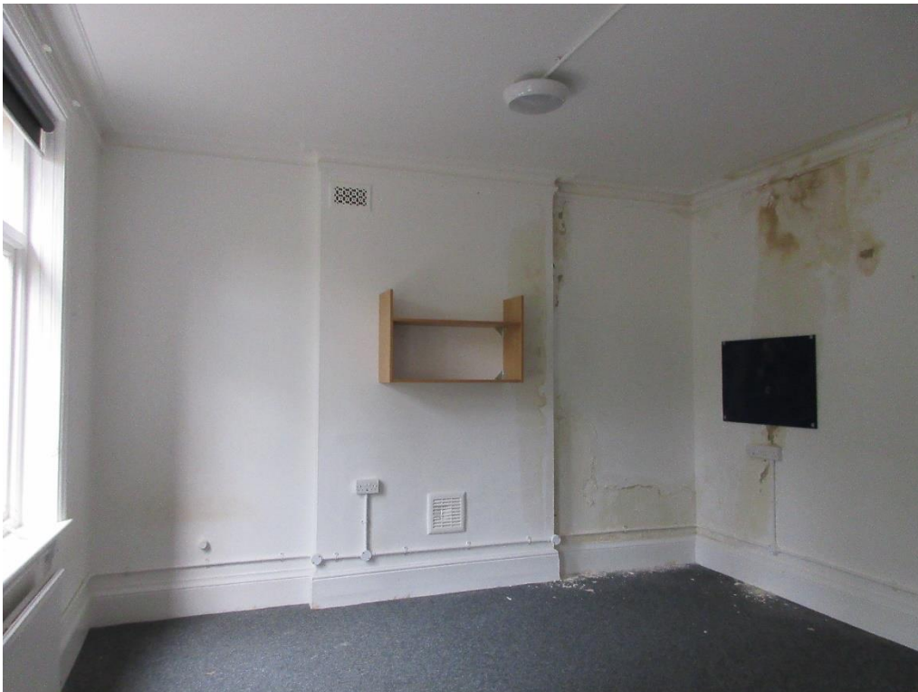
Figure 114: First floor of Red House – South-west room. Note original skirting, cornicing and chimney breast. Windows may be modern replacements. Note also unsightly wiring.
