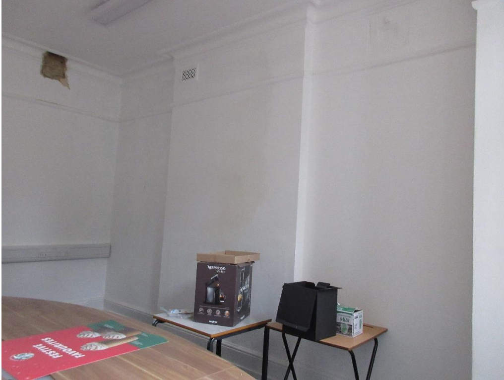
Figure 107: Ground floor of Red House – South-east room. Note original skirting, cornicing and picture railing, and chimney breast.
