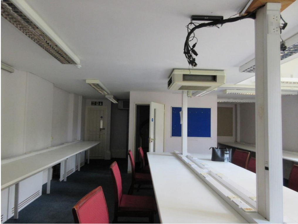
Figure 17: Ground floor – One of the rooms accessed from the north-west corridor, with its ceiling lowered by the mezzanine floor. Note modern partition walling around original fireplace and modern spiral staircase (see Figure 18).
