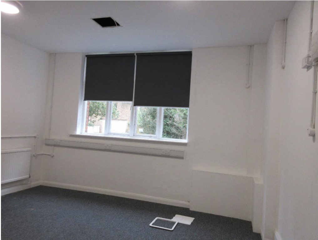
Figure 111: Ground floor of Red House – North-west room. Note modern lowered ceiling, modern skirting, and unsightly modern wiring and boxing-in.
