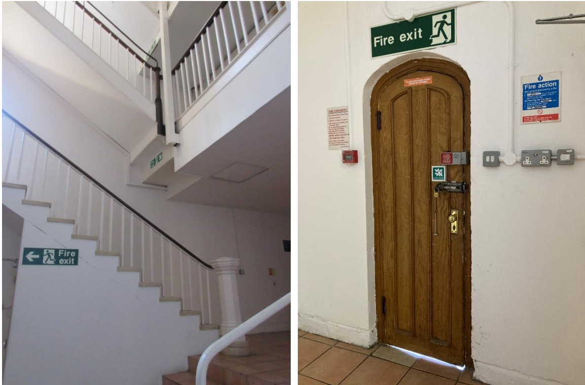
Figure 37 (left): Main staircase/landing by the south wing. Note newel post, balustrading and handrailing. This is the location of the proposed disability lift.
