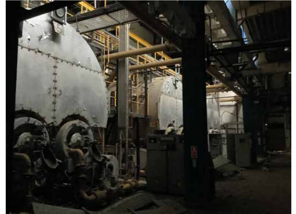
Remaining boiler tanks at ground floor in Energy Centre
