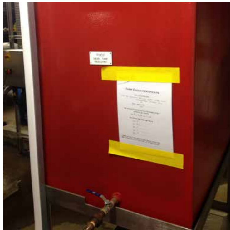
Decommissioned diesel tank in Production Office basement
