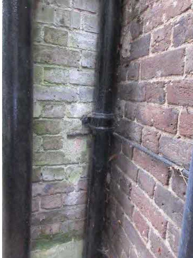
Figure 146: Side (north) elevation – join between rear and front parts. Note the misalignment of the brick courses.
