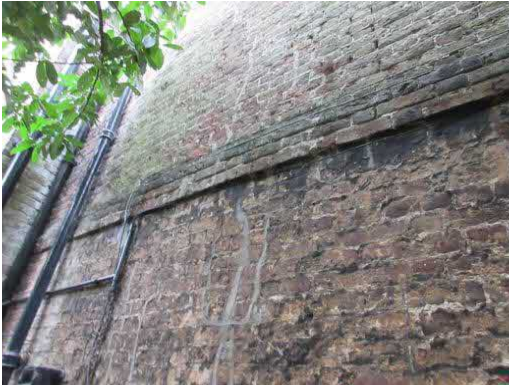
Figure 148: Side (north) elevation – front part. Note brick coursing, which is similar to that of the rear elevation.
