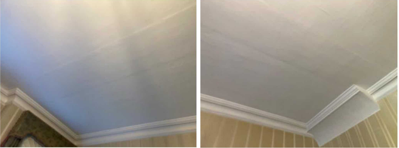
Figure 96 (left): Ground floor – scarring on ceiling in rear sitting room, where partition wall between rear sitting room and corridor used to be prior to 1968.
