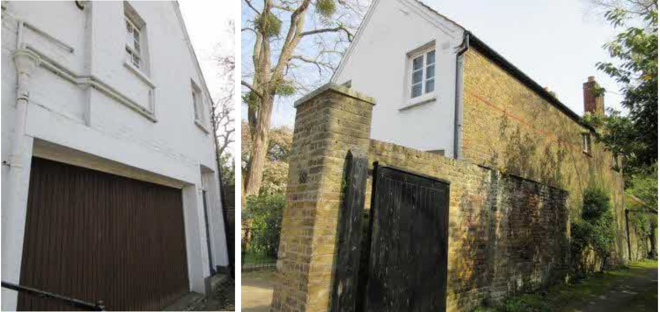
Figure 42 (left): Front elevation of garage (Flat 90B above), with garage door and door to Flat 90B (See also Figure 82.)
