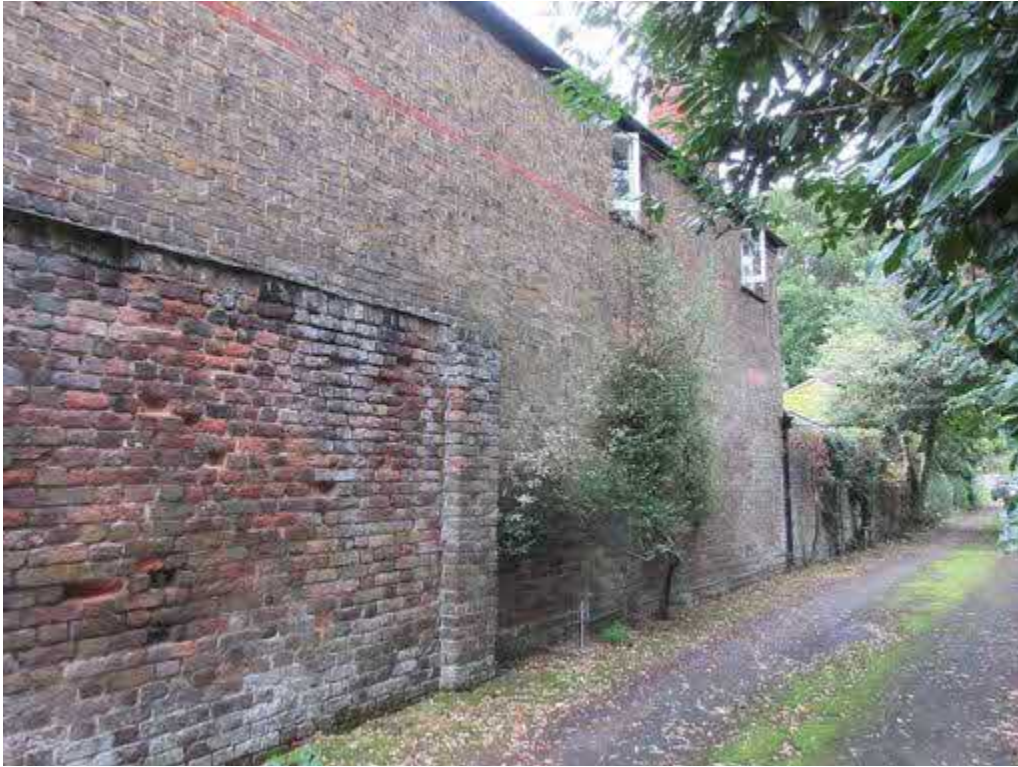
Figure 67: South elevation of house and boundary wall, seen from driveway to no. 88 Park Close. Note brick arches over bricked up window at ground floor level (where the existing stable is), and the chimney stack.
