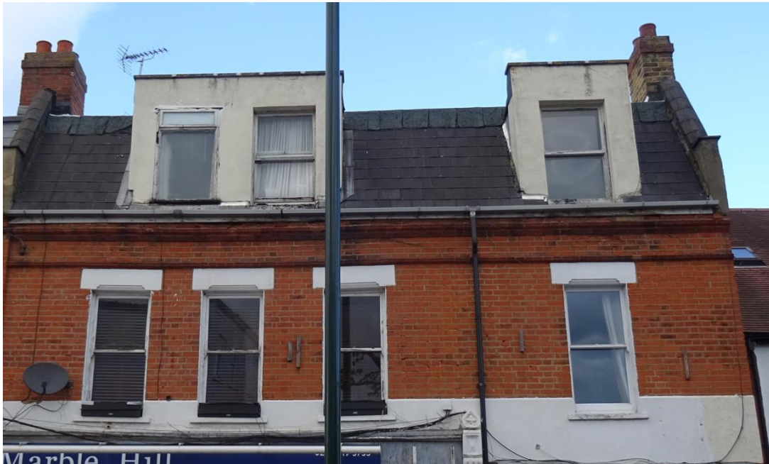
Fig 2: General view of the front elevation, showing the seven timber windows to be replaced
