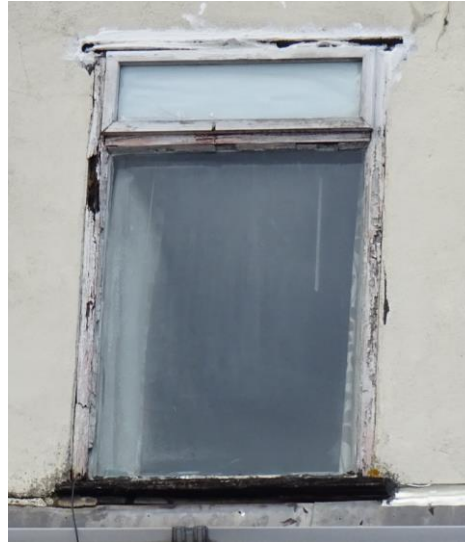
Fig 5: View of the existing top-hung casement and fixed pane window to the top floor front elevation, in dire need of replacement, and at odds with the sash windows elsewhere
