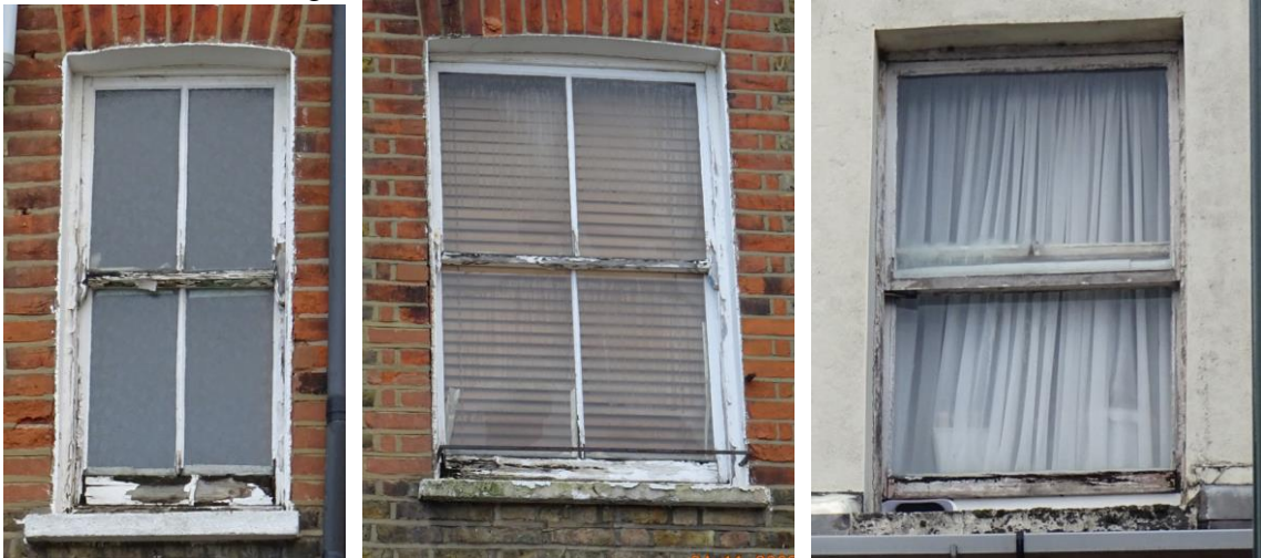
Fig 4: Views of the existing heavily degraded timber windows at the rear (left, centre) and front (right). Note also the absence of any “horns” to the window on the right.
