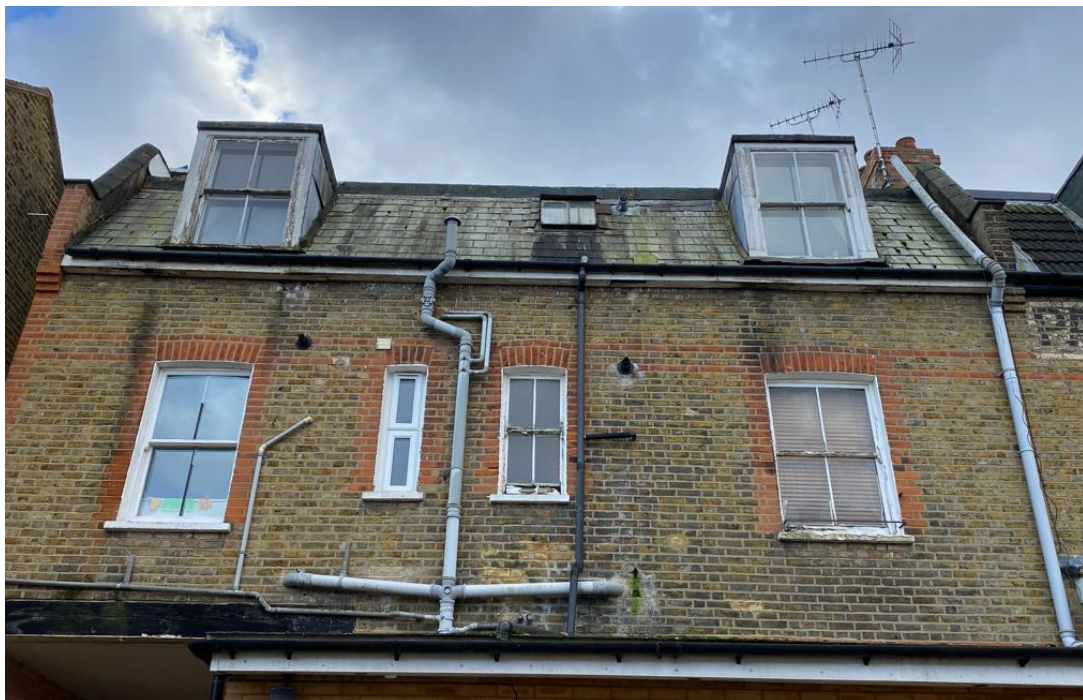
Fig 3: General view of the rear elevation, showing the six timber windows to be replaced, and one to be retained
