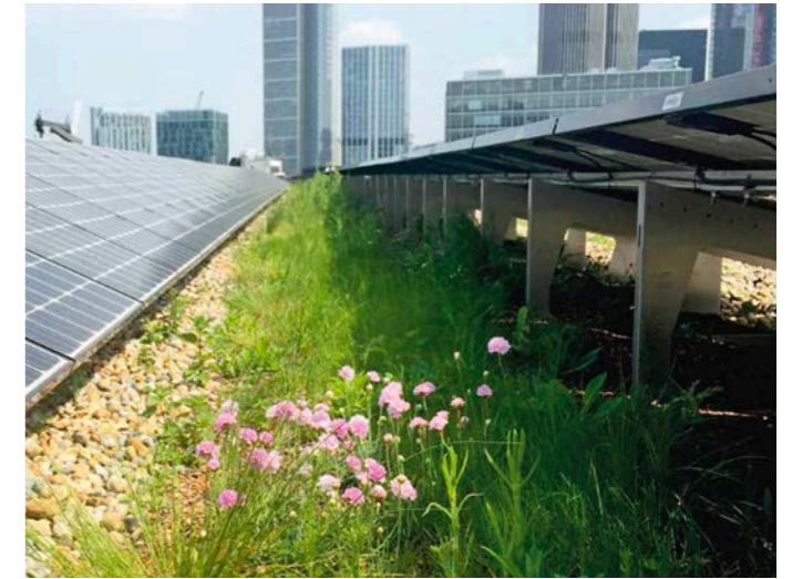
Photovoltaic Panels on Green Roofs
