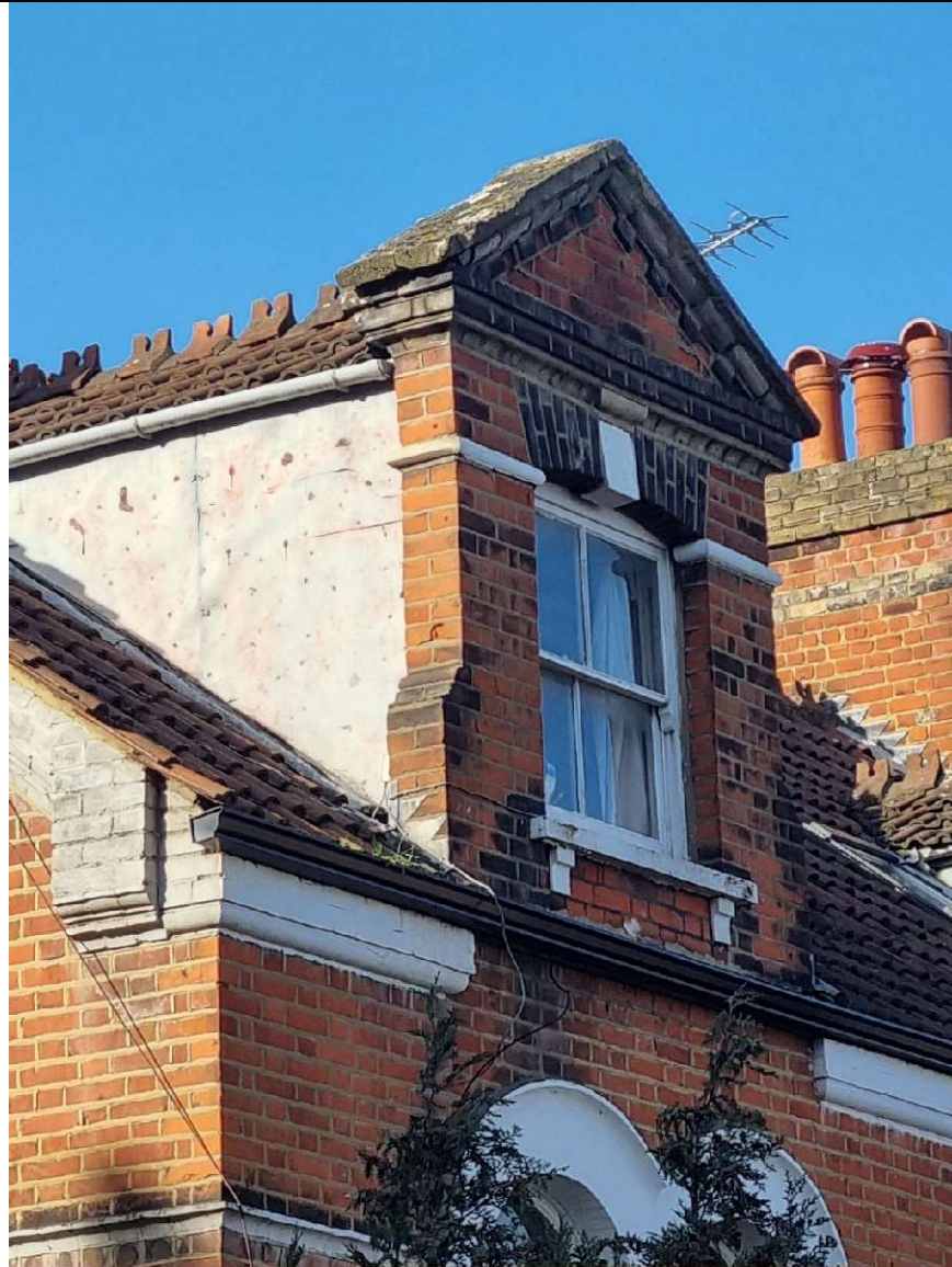
5.6 Stone corbel and string detail to be incorporated within the new proposal.
