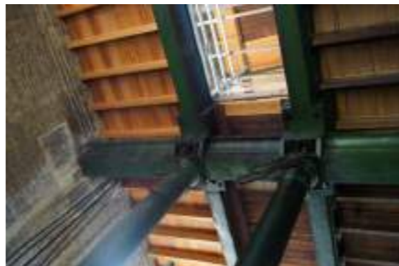
Tuscan order steel columns hold up the second floor's large steel beams in The Beam, Karslake
