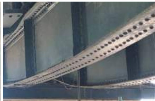
Large steel gantry crane at the top of the western pump house
