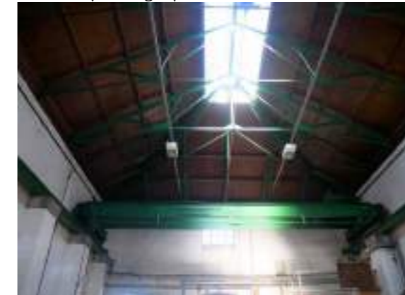
Workshop interior with glazed roof light in the southeast part of the building
