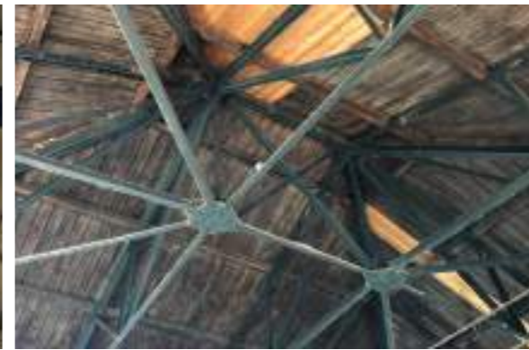
Intricate wrought iron truss work holds up the timber and slate roofs
