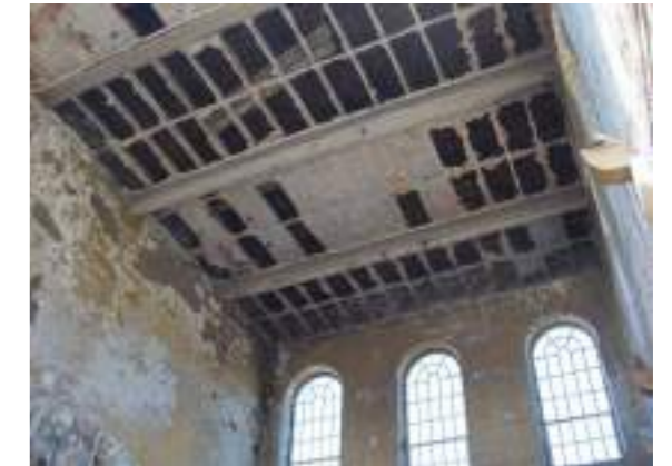
The western pump house is completely derelict and significantly deteriorating
