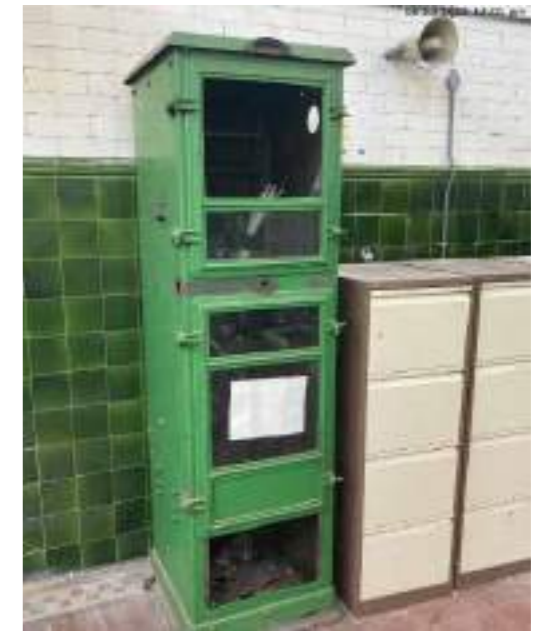
Harland control cabinet for electric centrifugal pump Date: 1932 Size: 0.6m x 0.6m Single Leaf Report comment: Low to medium significance
