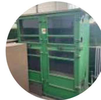
Item 6 Harland control cabinet for electric centrifugal pump Low to medium significance
