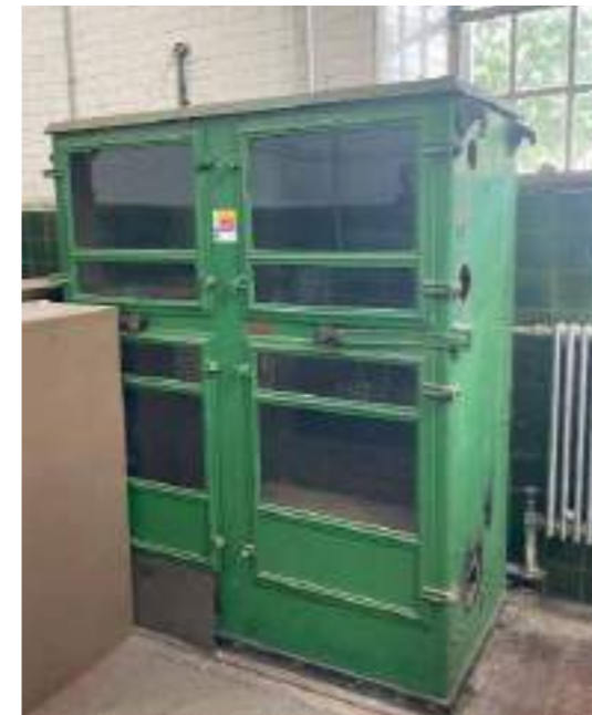
Harland control cabinet for electric centrifugal pump Date: 1932 Size: 0.9m x 1.7m Double leaf. Report comment: Low to medium significance
