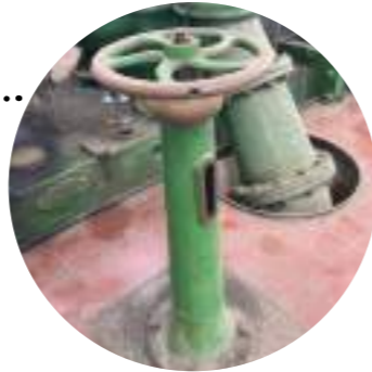
Item 9 Valve control standard for twin impellar electric centrifugal pump set Low to medium significance
