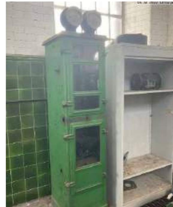
Harland control cabinet for electric centrifugal pump Date: 1932 Size: 0.5m x 0.5m Single Leaf Report comment: Low to medium significance
