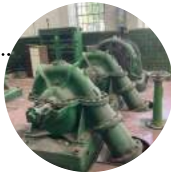
Item 4 Harland twin impellar electric centrifugal pump set Low to medium significance
