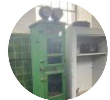
Item 8 Harland control cabinet for electric centrifugal pump Low to medium significance
