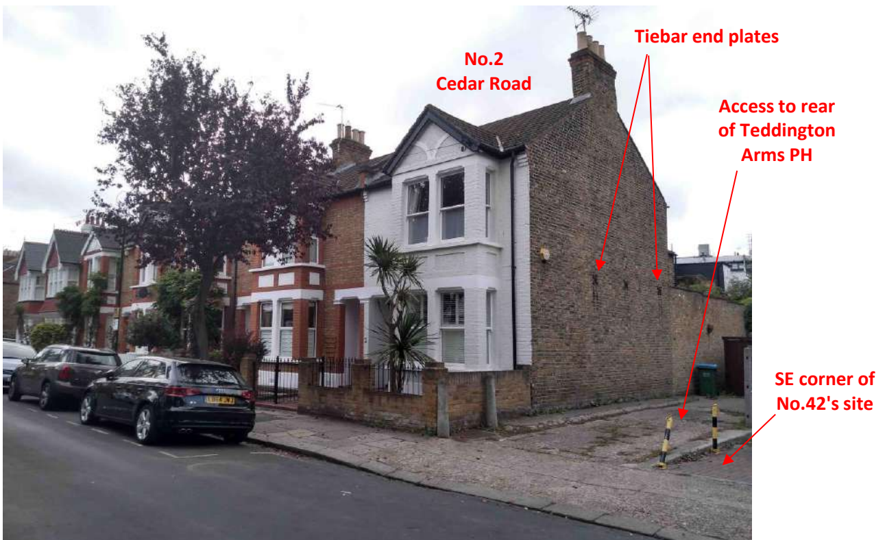
Photo 4: Terraced housing to rear of site. Tie bars supporting gable wall suggest that there has been past structural damage.
