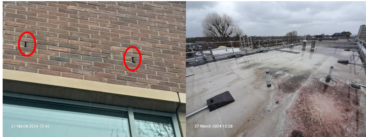
Gaps in the mortar which provide crevice habitat for bats (left) and the flat roof (right).
