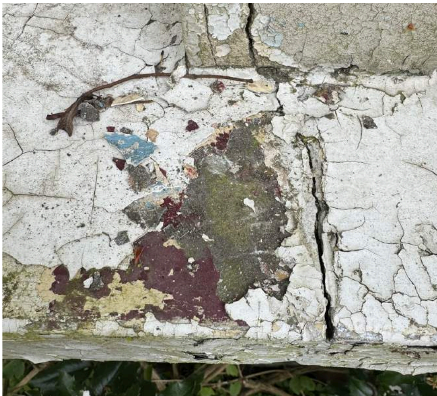
The poor condition of the existing masonry due to years of neglect and water damage caused by overpainting
