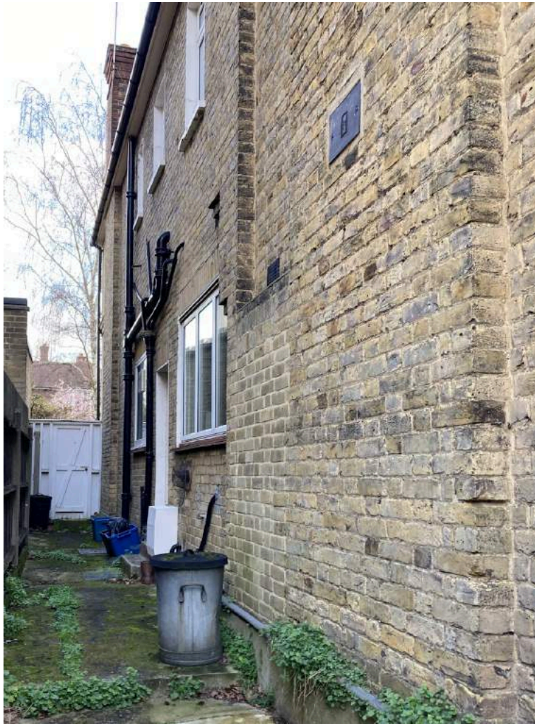
The poor quality north-west elevation which is proposed to be insulated
