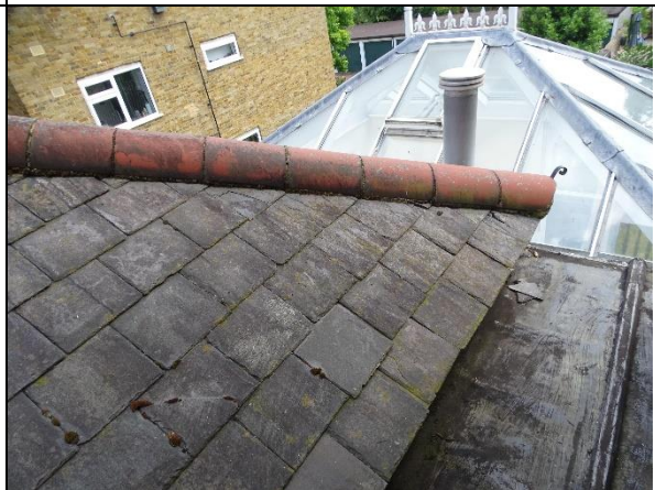
Photo 10: View of former coach house roof with glass conservatory roof to the rear
