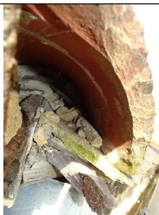
Photo 14: View into circular ridge tile showing lack of access beyond concrete plug
