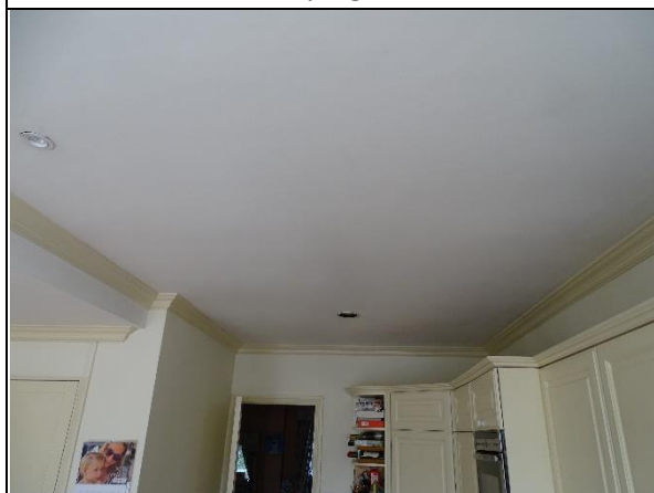
Photo 15: Kitchen ceiling within the ground floor of the former coach house within no access to roof void via the ceiling
