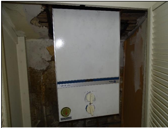
Photo 7: Disused boiler in cupboard abutting main roof
