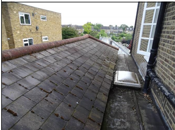
Photo 11: Sealed brick tile ridge and slate tile roof of former coach house
