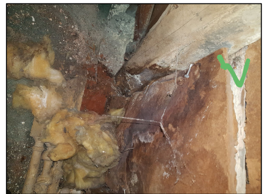
Picture taken in the roof void. Some of the bearing ends of the rafters are rotten/decayed and need to be supported.
