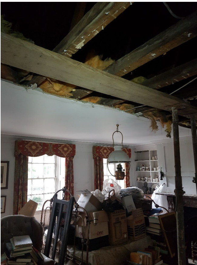
Left: The second floor ceiling has collapsed.
