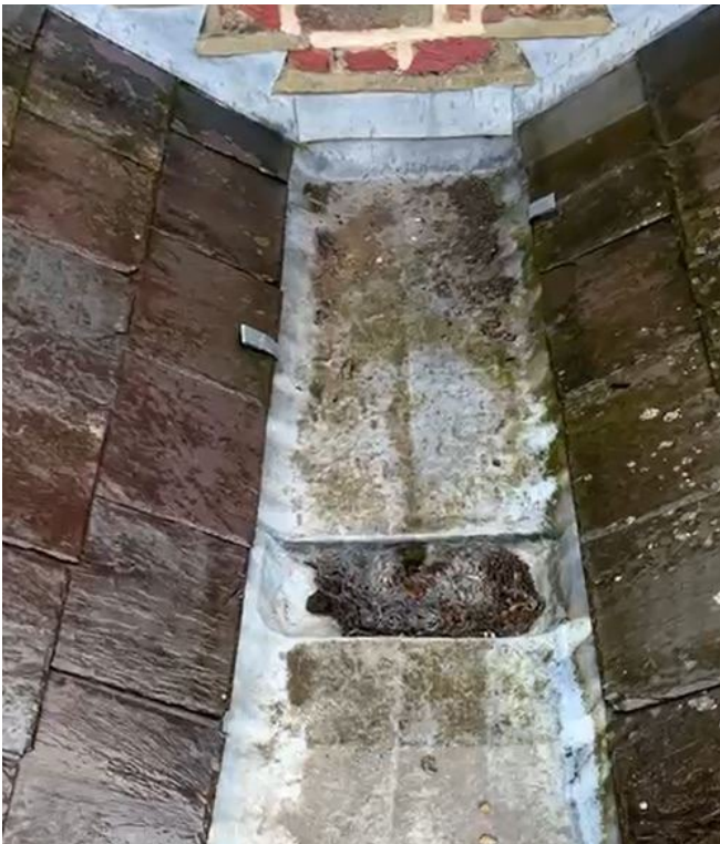
Above Left: The valley has a gully at its southern end that connects into an open timber chute within the attic space and the rear closet wing roof and out to its rainwater hopper and downpipe. We would like to retain this chute for historical value but install a drainage pipe within it to ensure drainage is robust.
