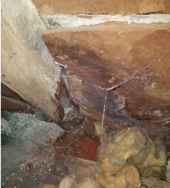
Left: Picture taken in the roof void. Some of the bearing ends of the rafters are rotten/decayed and need to be supported.
