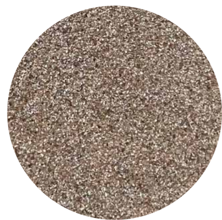
Existing Pebble Dash Render stripped back to block work behind
