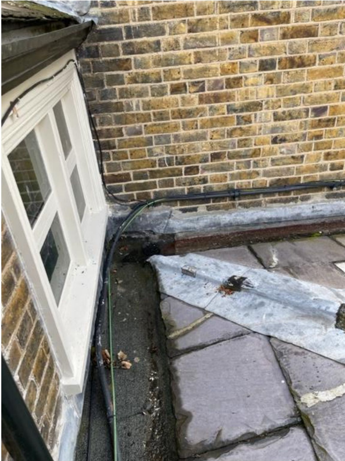
Photo 6 Rainwater gutter above defective roof timbers
