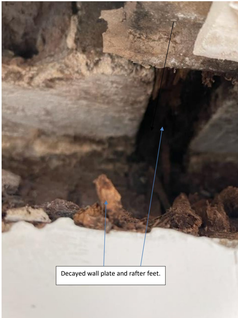
Photo 2 Close-up of decayed timbers
