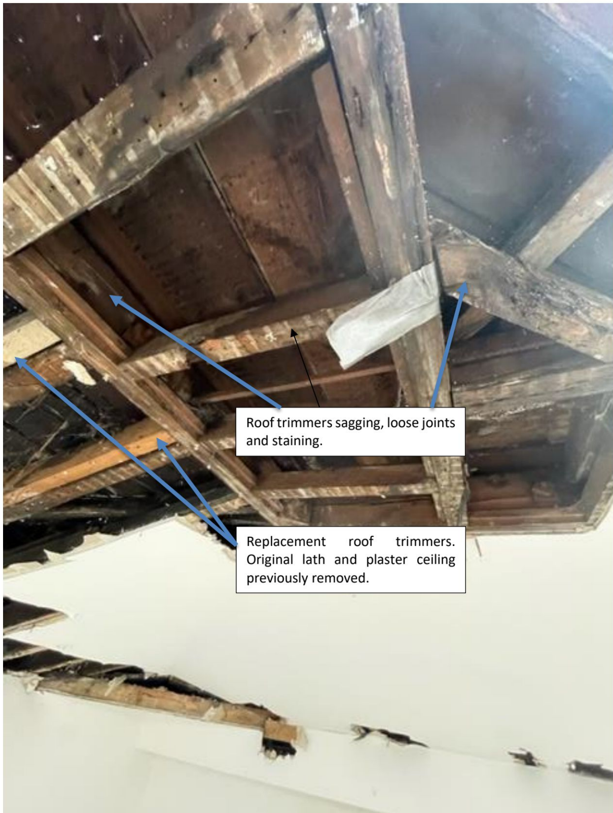
Photo 4 Poor condition of roof timbers
