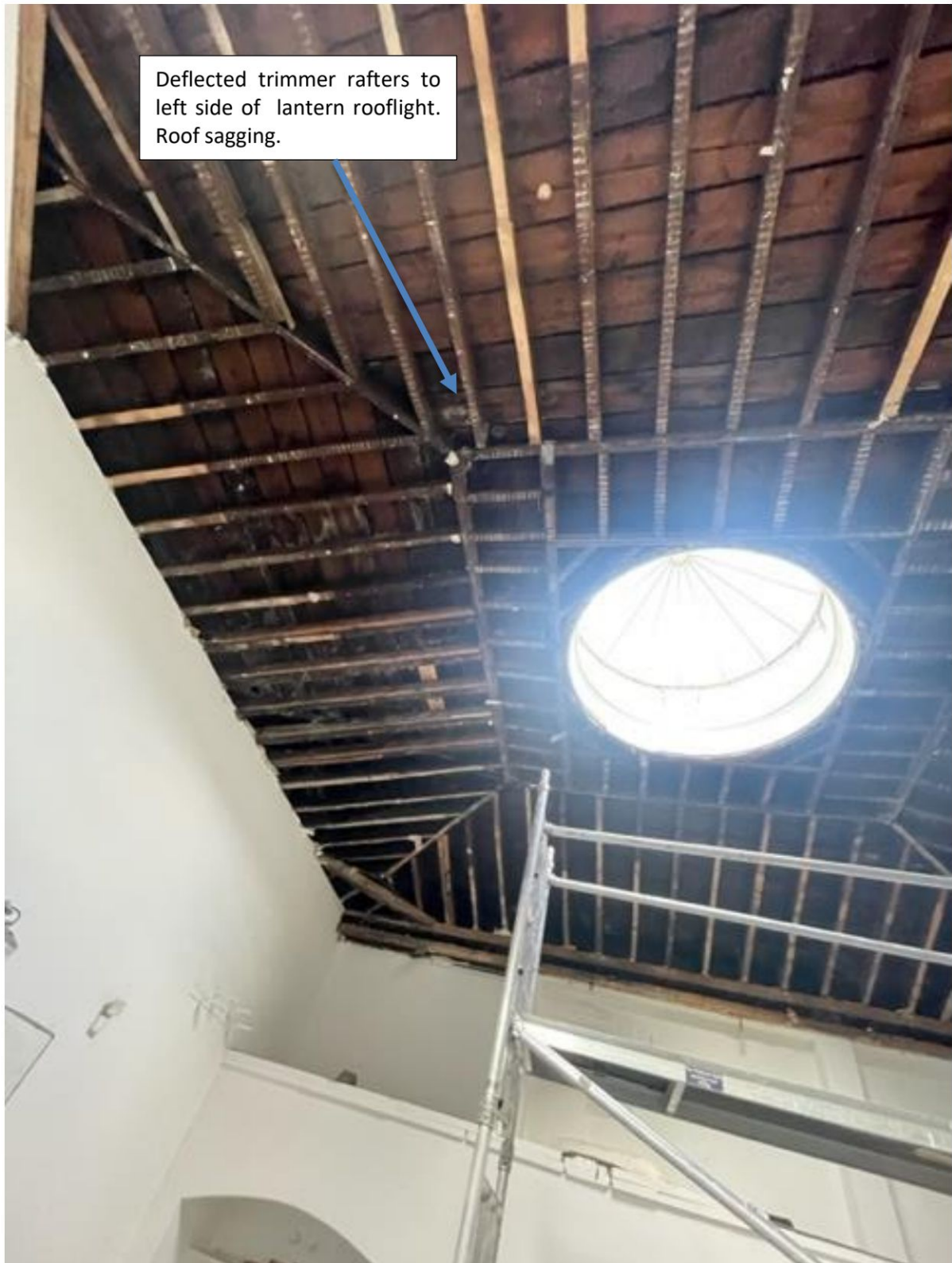
Photo 2 Sagging roof trimmers around rooflight
