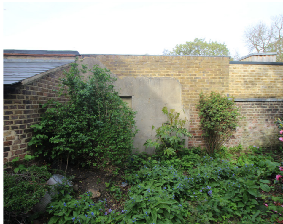
Fig 8. Photo 5. - Tall boundary wall between no. 7 & no. 9. A mixture of differing constructions.
