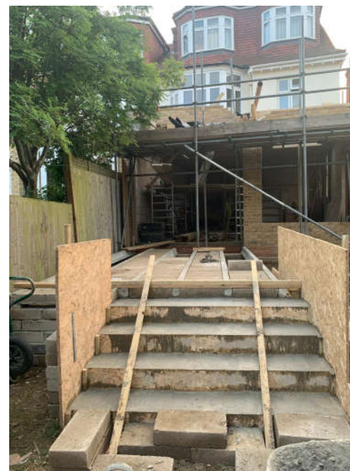
Patio constructed using approved beam and block method to span over Rowan tree 5 July 2023
