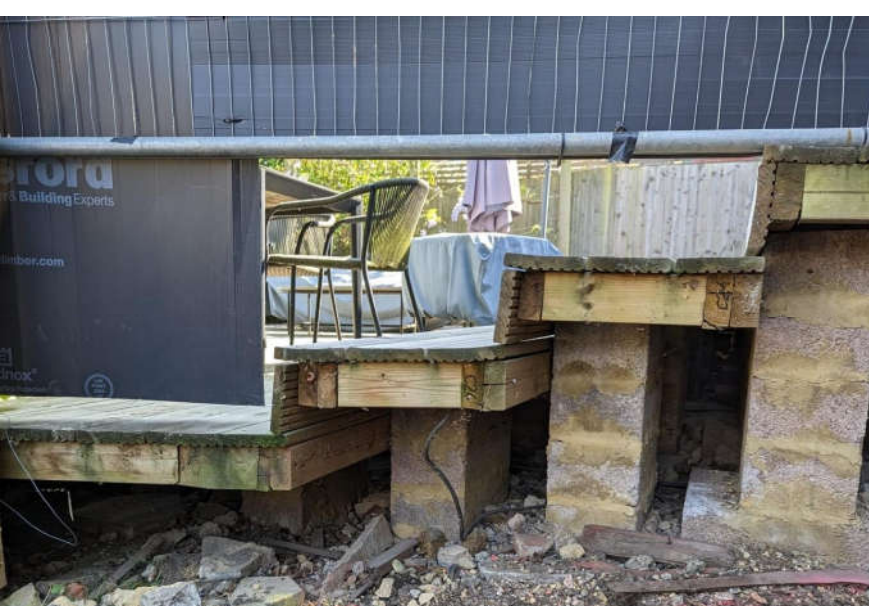
Rowan tree roots are constricted under neighbours' concrete blocks and decking at no. 203. 25 May 2023
