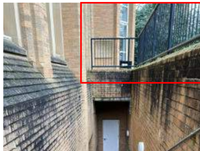
Sir Cyril Taylor Library - existing balustrade to be matched
