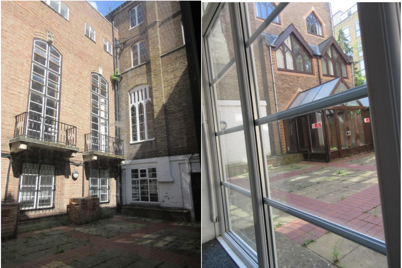
Figure 17 (left): South-east elevation of rear extension A, and south-west elevation of the principal building.
