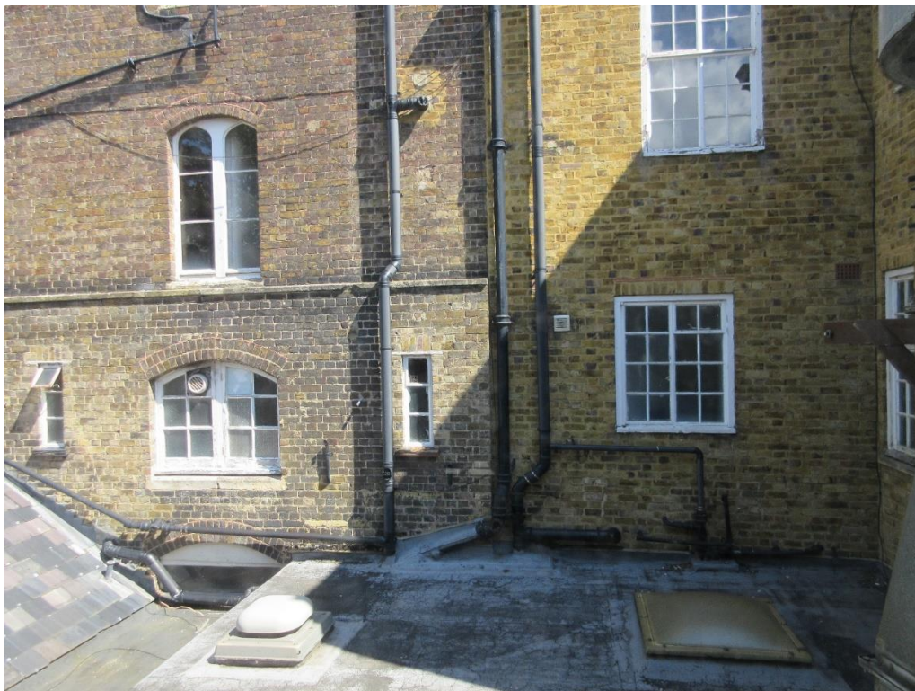
Figure 22: Rear of the principal building on the left, and rear of George House on the right (viewed from extension E).
