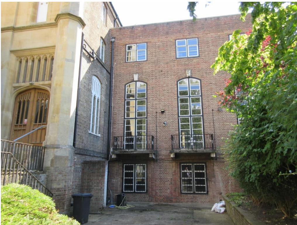
Figure 16: North-west elevation of north wing of the principal building and a glimpse of its rear (south-west) elevation, and the north-west elevation of rear extension A.
