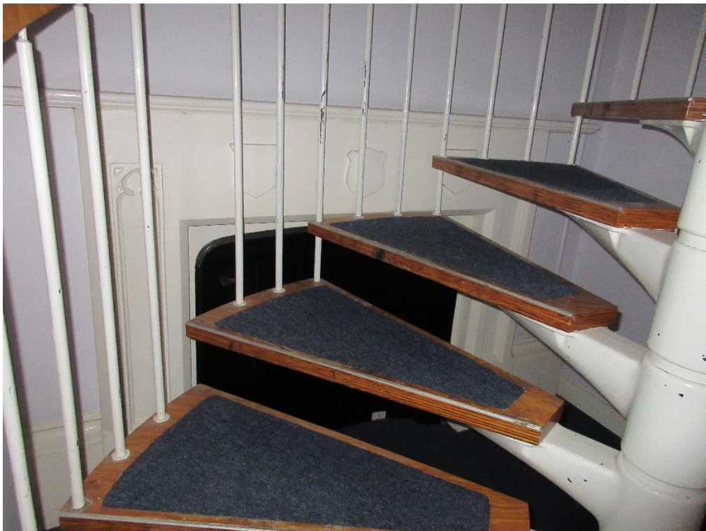
Figure 60: Modern spiral staircase (which leads to the mezzanine floor) and original fireplace, in ground floor room accessed from the north-west corridor (see Figure 59). Consented application ref: 24/0524/LBC involved the removal of this staircase.
