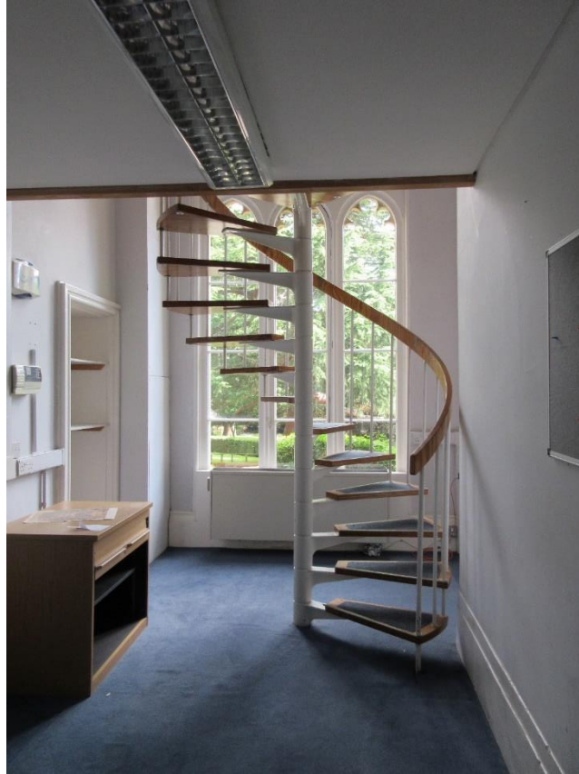
Figure 61: Modern spiral staircase (which leads to mezzanine floor). Current application involves the removal of this staircase, and the ceiling/mezzanine floor.
