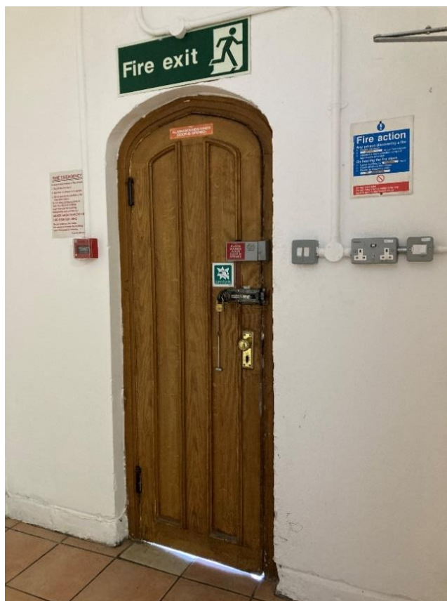
Figure 64: Interior of side entrance door to south-east elevation. (See Figure 67 for the exterior of the door.)
