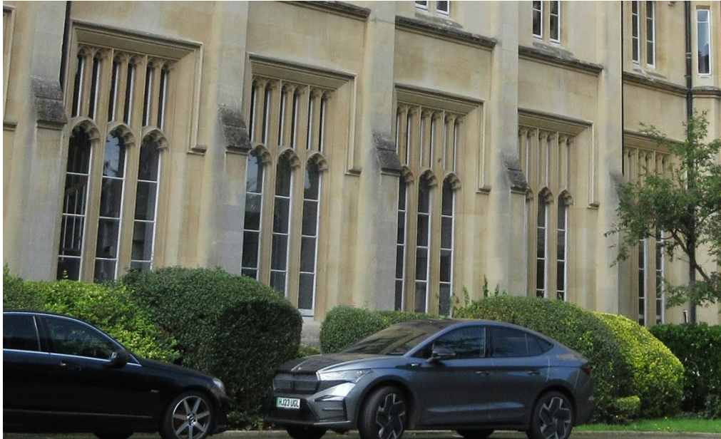
Figure 75: Front (north-east) elevation of principal college building – to the north of the entrance, at ground floor level.
