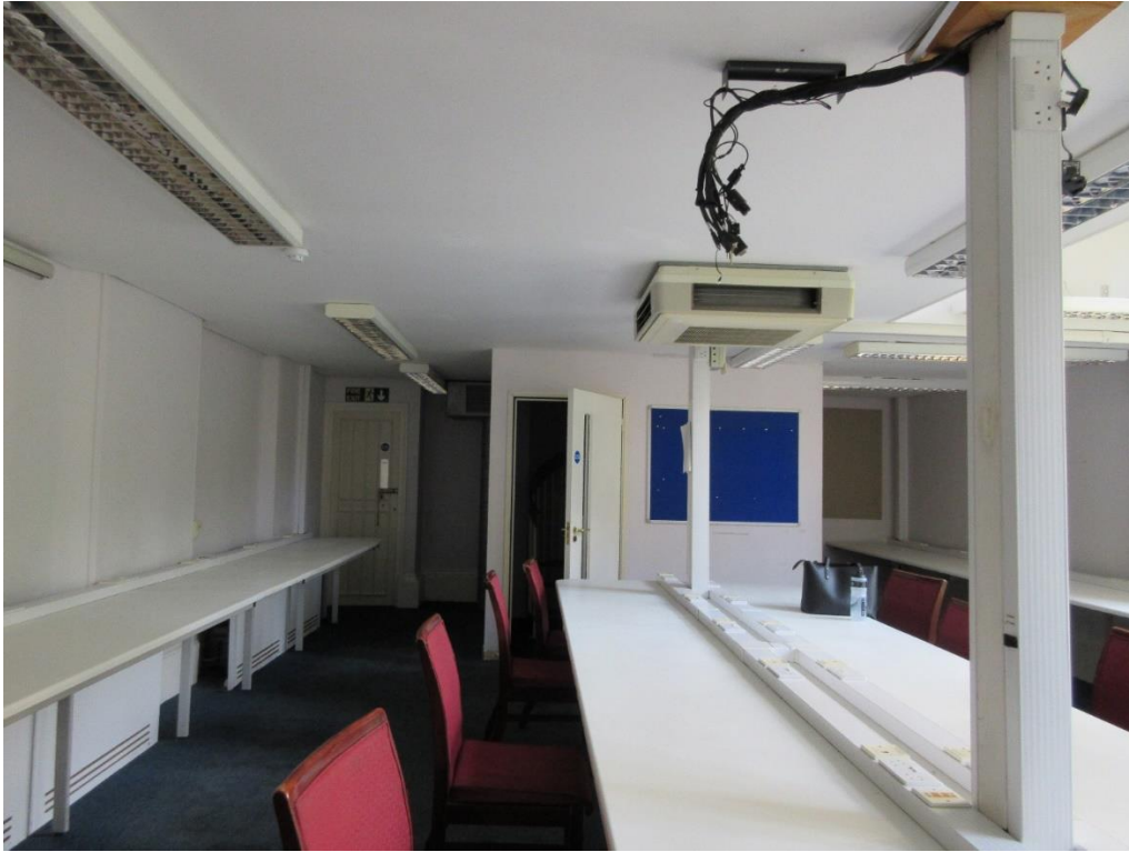
Figure 59: Ground floor – One of the rooms accessed from the north-west corridor, with its ceiling lowered by the mezzanine floor. Note modern partition walling around original fireplace and modern spiral staircase (see Figure 60). Consented application ref: 24/0524/LBC involved the removal of these walls. Current application involves the removal of the modern ceiling/mezzanine floor.
