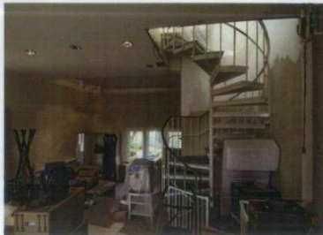
View of Living room with open spiral steel Stair to first floor. New stair will be dog- leg, and be in oak construction.
