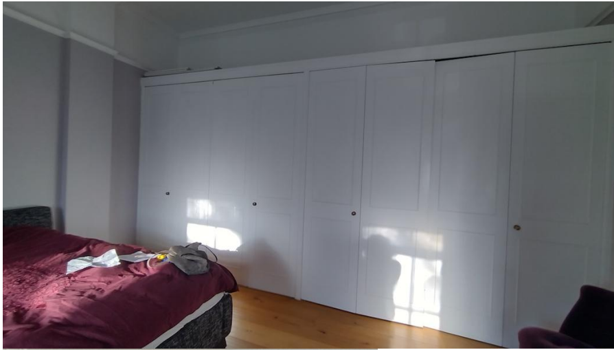
a.view towards the wardrobes in the main bedroom to be demolished. The joinery is constructed of door blanks with plant on moulding and brass knobs.
