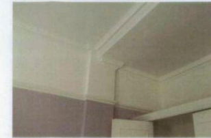
Typical 1st floor cornices. All ground and 1st floor cornices to remain.
