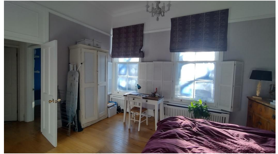
b.view towards the existing bedroom door that will be infilled. The front elevation is to remain as existing
