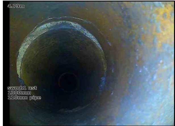
swmh1 ustX_744db1a9-66bf-4853-be06-8646d82032f3_20240207_221 800_805.jpg, 00:00:43, 4.79 m Crack, circumferential from 10 o'clock to 3 o'clock
