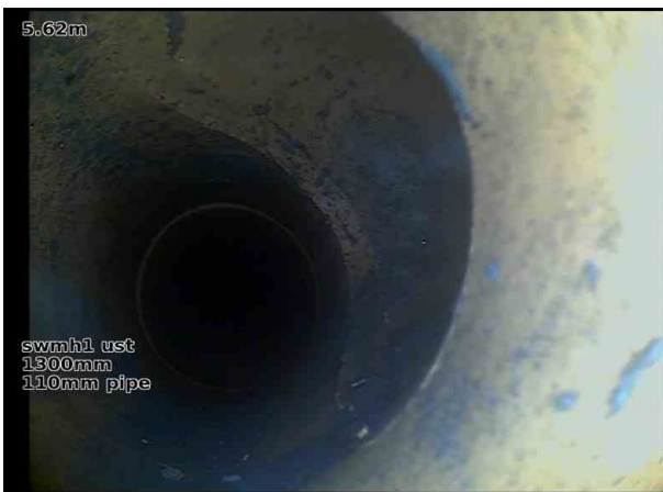
swmh1 ustX_ddc152bf-132d-4025-a85d-9dd618a7cd65_20240207_22 2312_190.jpg, 00:01:01, 5.62 m Junction at 3 o'clock, diameter: 100mm, RW GULLY FRONT
