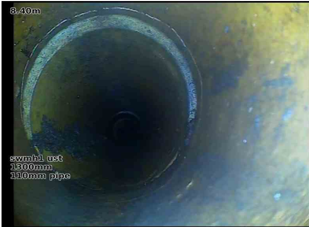
swmh1 ustX_88fb792e-55b9-48ef-bc98-570d9852f815_20240207_222 441_859.jpg, 00:01:31, 8.40 m Crack, circumferential from 9 o'clock to 4 o'clock
