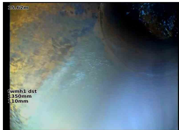
fwmh1 ustX_f3409cce-d124-43a1-8347-99480b4b0e70_20240207_225 539_679.jpg, 00:02:27, 15.62 m Line deviates right, full
