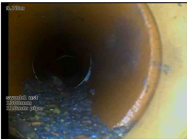
swmh1 ustX_234c706c-b2e1-4624-b9bc-79ff22d21aa0_20240207_222 604_259.jpg, 00:01:49, 9.73 m Settled deposits, coarse, 25% cross-sectional area loss, start
