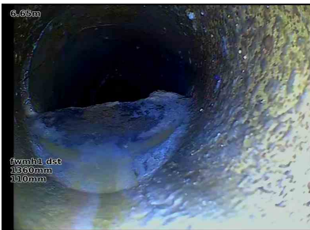
fwmh1 dstX_83d30b6c-5624-4347-8e81-75e390a2cda4_20240207_22 3828_574.jpg, 00:00:41, 6.65 m Attached deposits, encrustation from 4 o'clock to 8 o'clock, 40% cross-sectional area loss
