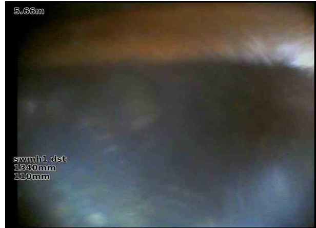
swmh1 dstX_89510f10-b9d5-4fd2-bedd-96ab472e9c7a_20240207_223 305_472.jpg, 00:00:55, 5.66 m Finish node, major connection without manhole, reference: sewer
