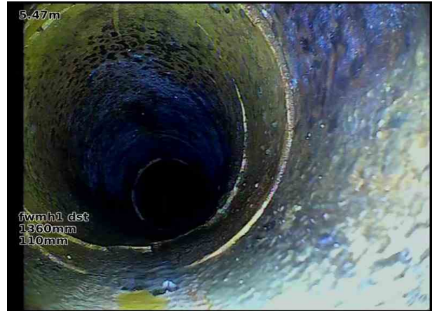
fwmh1 dstX_096bf927-93a1-4fe4-b8ad-7e2d9b055c24_20240207_223 712_243.jpg, 00:00:34, 5.47 m Fracture, circumferential from 3 o'clock to 7 o'clock
