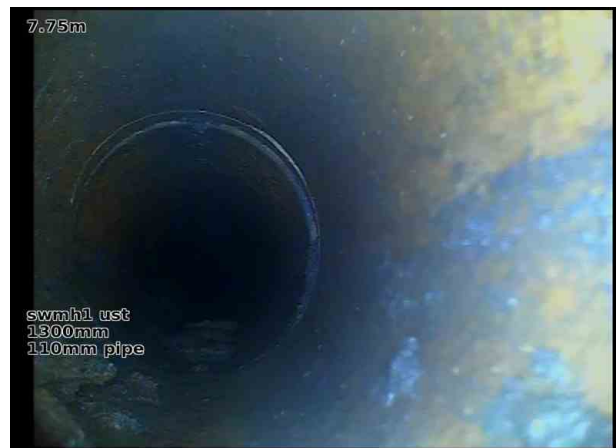
swmh1 ustX_9934facb-32d6-4f6c-9b6a-c3d7c3e11067_20240207_222 401_502.jpg, 00:01:23, 7.75 m Crack, circumferential from 9 o'clock to 2 o'clock
