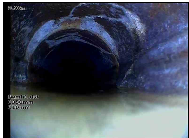
fwmh1 ustX_470b1b70-0fa4-41ef-996a-31671add2df9_20240207_225 139_933.jpg, 00:01:21, 9.96 m Cracks, multiple from 11 o'clock to 2 o'clock
