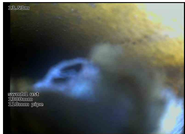
swmh1 ustX_ea60d295-071d-4961-abab-0d2ce511bfaa_20240207_222 849_671.jpg, 00:02:22, 13.53 m Settled deposits, coarse, 60% cross-sectional area loss, finish
