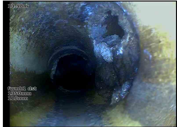
fwmh1 ustX_6f7f92c5-4e28-4a54-a6c5-e3c877256071_20240207_225 328_659.jpg, 00:01:57, 13.98 m Junction at 3 o'clock, diameter: 100mm, Redundant junction
