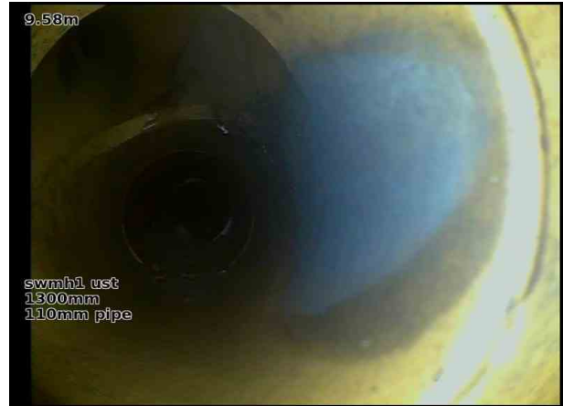
swmh1 ustX_0260c911-b0a5-43b6-a559-8199e072db75_20240207_22 2522_039.jpg, 00:01:42, 9.58 m Junction at 12 o'clock, diameter: 100mm
