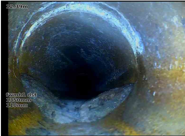
fwmh1 ustX_77720550-3be4-41dc-984a-ca4aefc549b7_20240207_225 230_182.jpg, 00:01:44, 12.39 m Crack, circumferential from 9 o'clock to 3 o'clock
