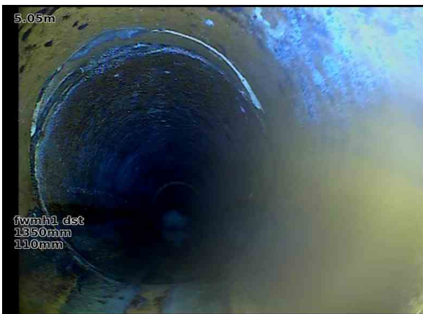
fwmh1 ustX_b9be31e4-d4da-4770-a288-e532082d8efe_20240207_224 342_831.jpg, 00:00:36, 5.05 m Crack, circumferential from 9 o'clock to 2 o'clock
