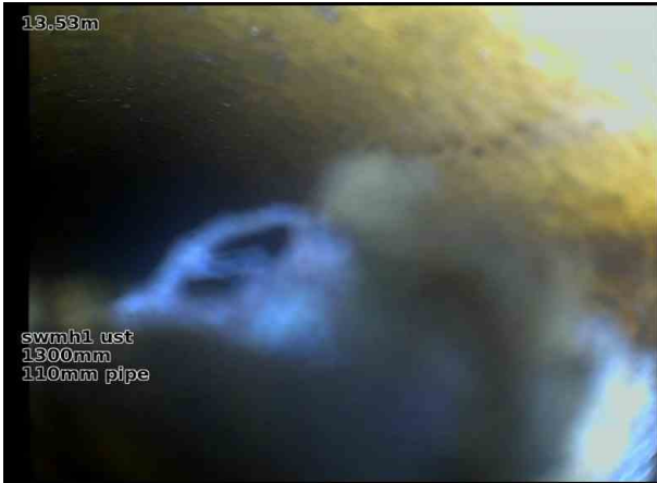
swmh1 ustX_6634cadc-a9b0-4104-a63f-66d5dcec7ec6_20240207_222 929_225.jpg, 00:02:22, 13.53 m Survey abandoned, Survey abandoned due settled deposits coarse in the pipe
