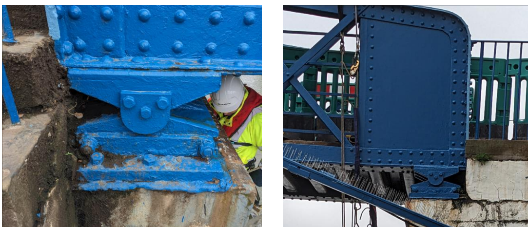
Figure 2. Left photo: bearing under west girder. Right photo: bearing under east girder
