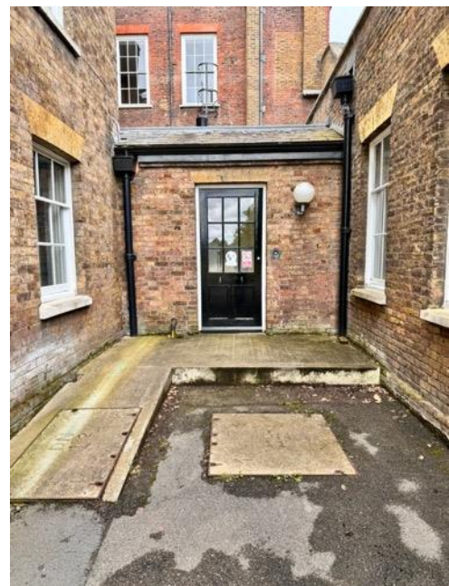
Existing Annex Door with no access control externally. NB this is the only wheelchair access but note the ramp is not compliant with current regulations.
