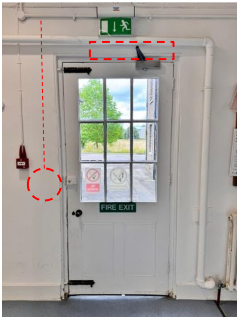
Existing annex door – proposed locations of access controls and automatic overhead door opener
