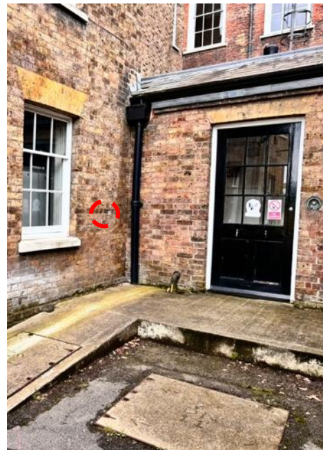
Existing annex door – proposed location of external fob (no external cabling required)
