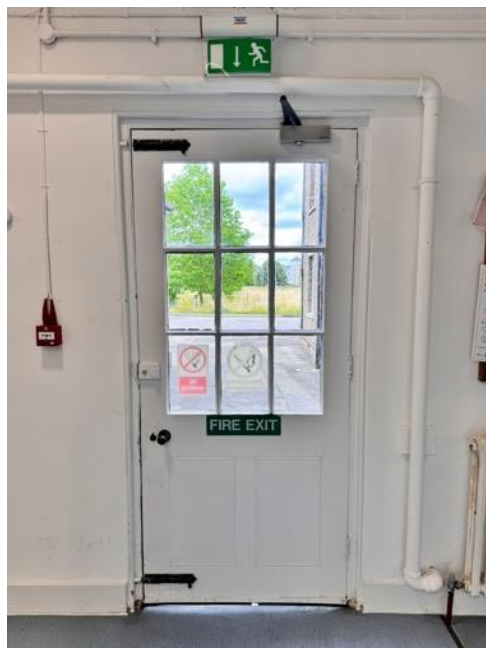
Existing Annex Door with no access control internally
