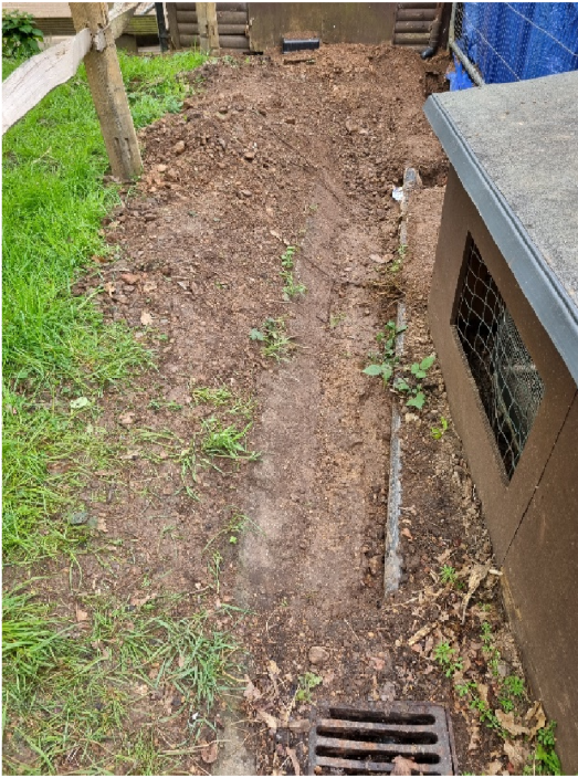
Figure 7: Uncovered concrete to the north of the kerb.
