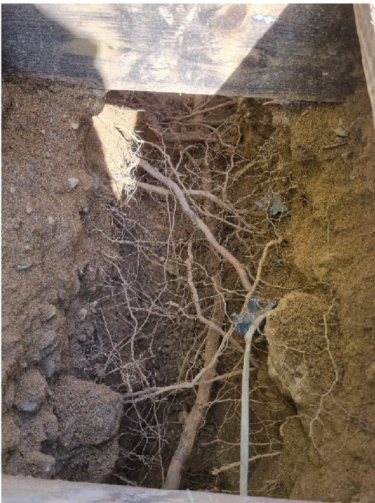
Figure 5: Numerous oak roots uncovered from T45 before pruning.
