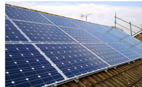
Figure 6 – Roof mounted PV panels
