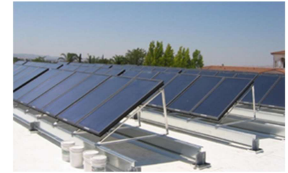
Figure 7 – Frame mounted PV on flat roof
