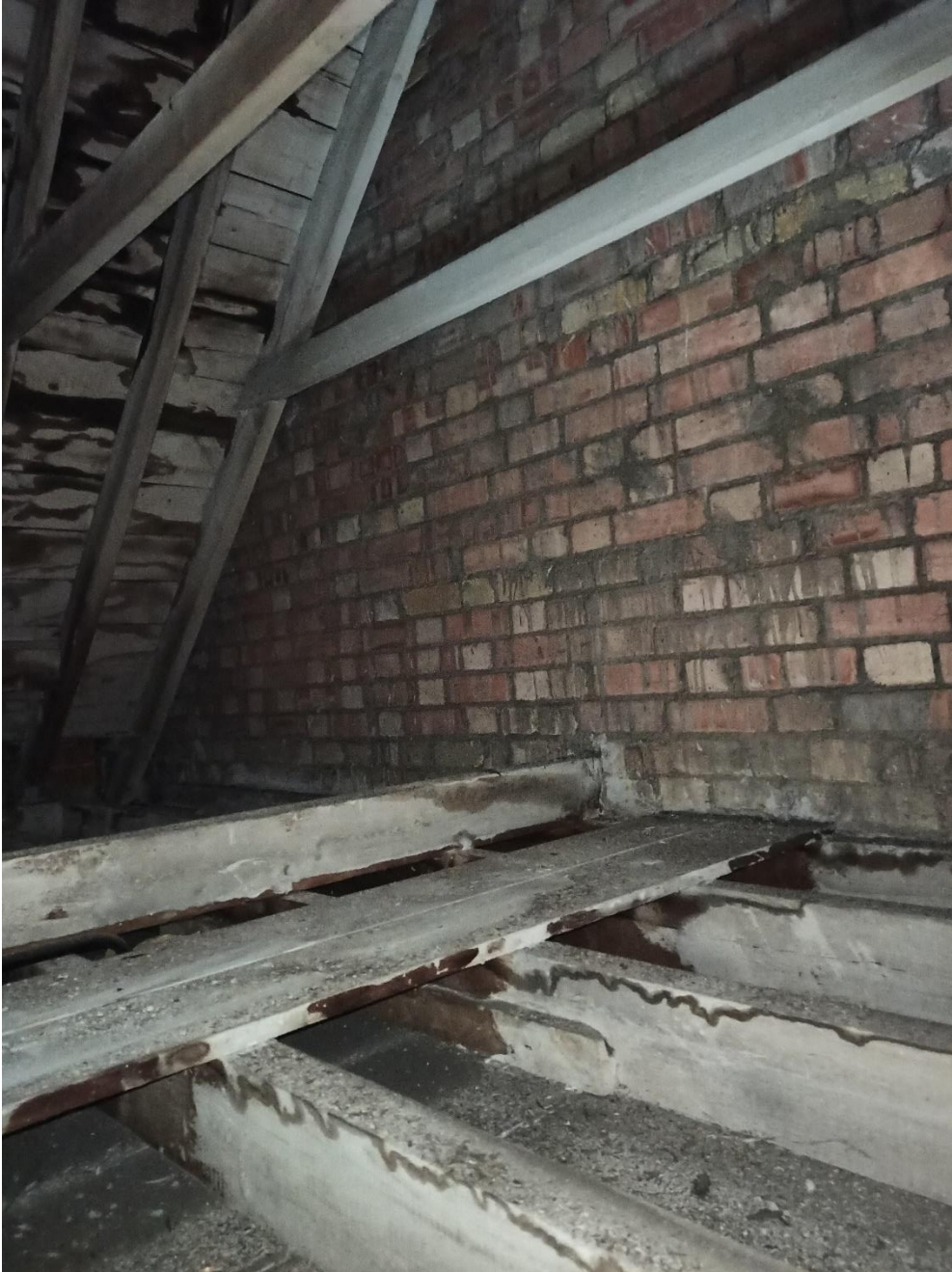
Photo 2 – Timber members forming roof showing water staining.
