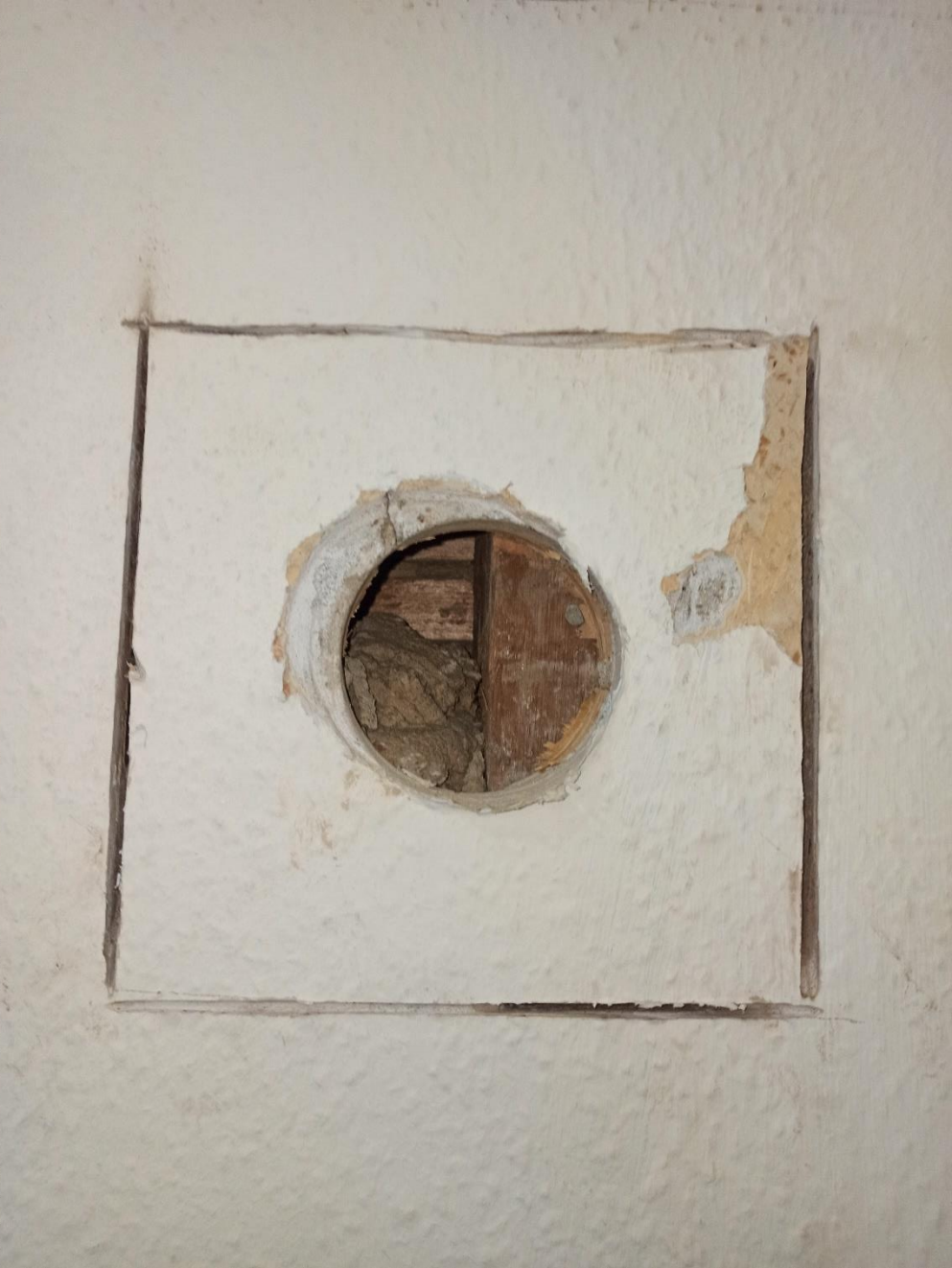
Photo 6 – Hole in wall indicating mortar render over timber studwork.
