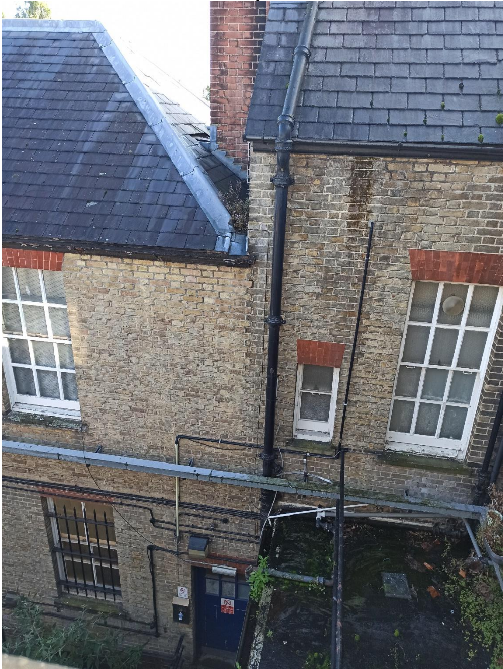
Photo 16 – Crack in external brick façade.
