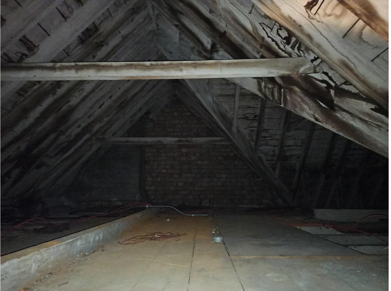
Photo 4 – Boarded out and staining to loft space and timber members in reasonable conditioning, but showing water damage.
