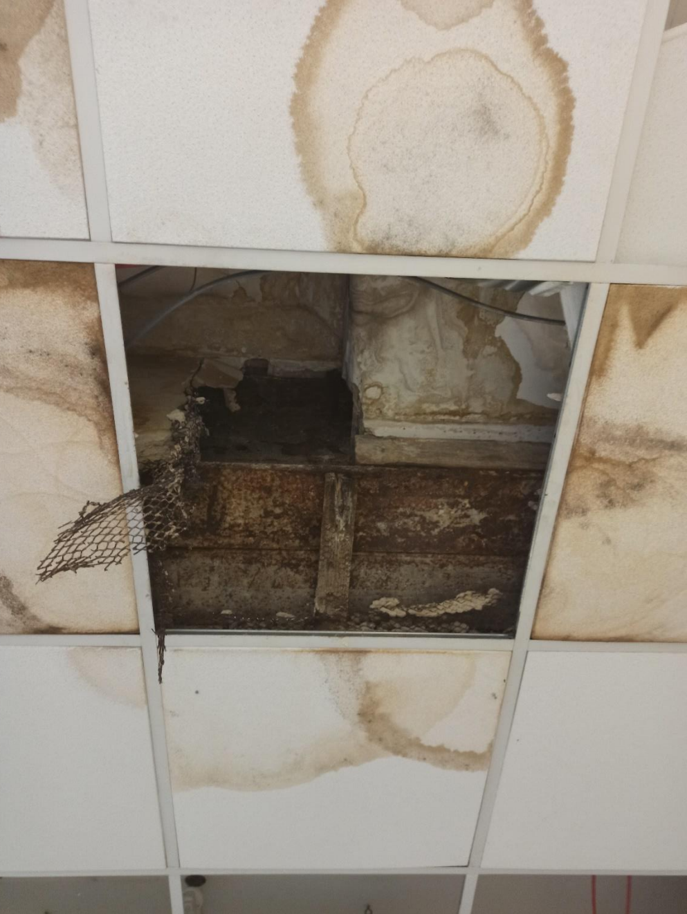
Photo 12 – Ceiling opened to show corroded steel beams.
