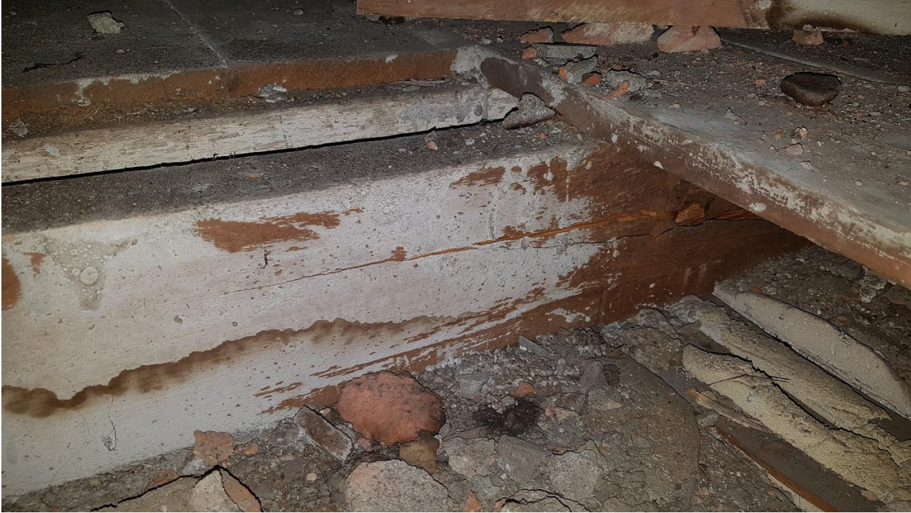
Photo 8 – Timber members showing splitting in centre.
