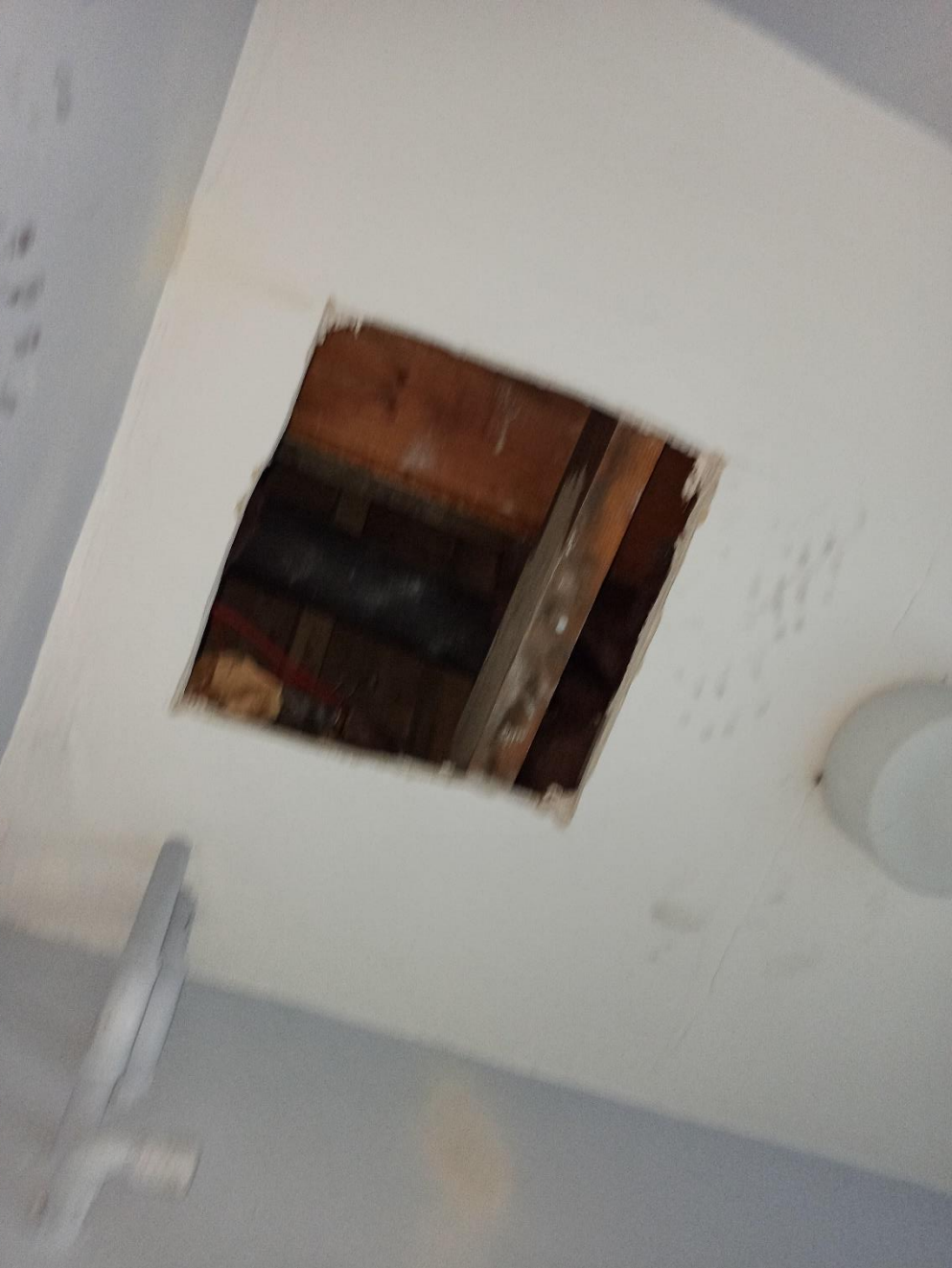
Photo 5 – Hole in ceiling indicating timber roof rafters in reasonable condition.
