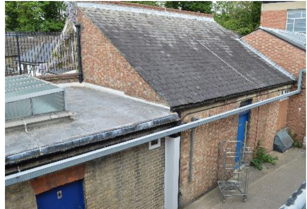
The 1930s link block (left) and the much-altered brick shed (right) of the western rear wing.
