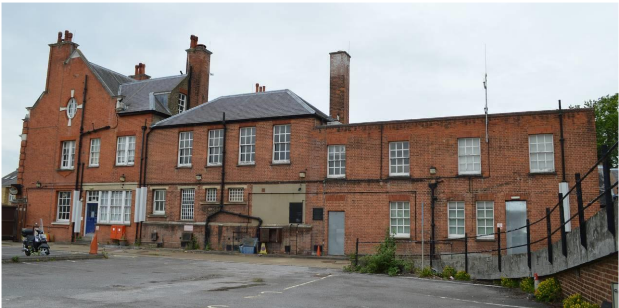
The east façade, showing the transition from the well-detailed gable by the road (left), to the plain rear wing (centre) and the 1930s flat-roofed extension (right).
