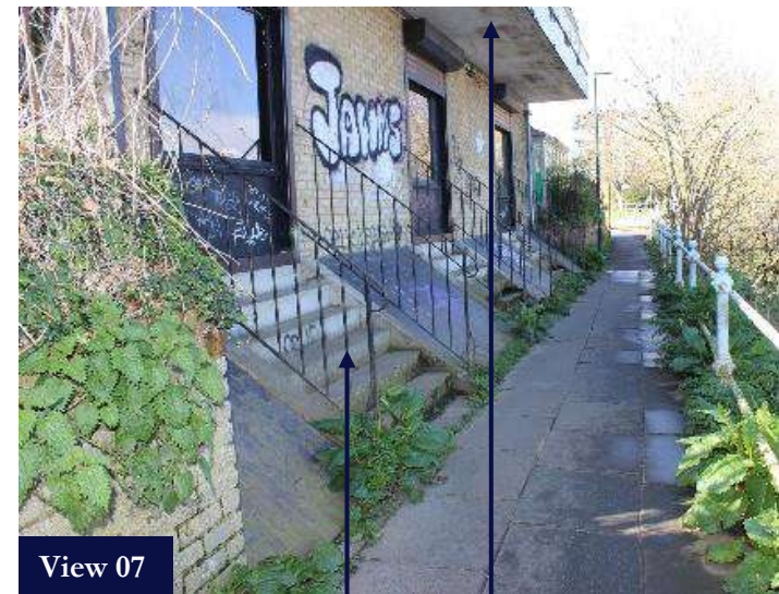
Area used by loiterers – Metropolitan Police support removal of canopy and steps to eradicate Anti-Social behaviour
