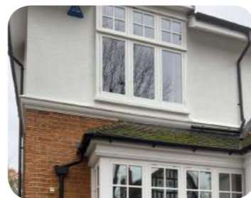
Painted timber window to ground floor north elevation to match the existing windows
