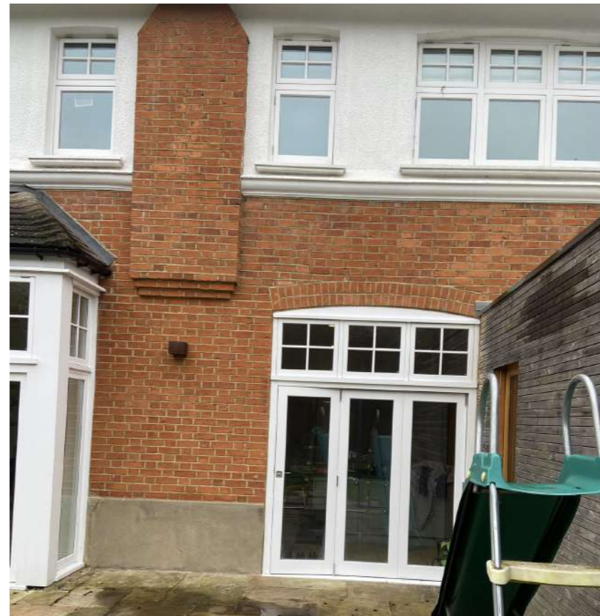
Existing bifold doors to the rear elevation are to be retained, with a new window proposed below the existing chimney breast.
