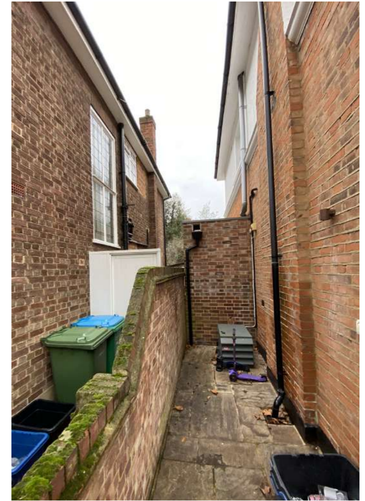
View from the west elevation towards the existing side extension alongside No.15 Cole Park Road.
