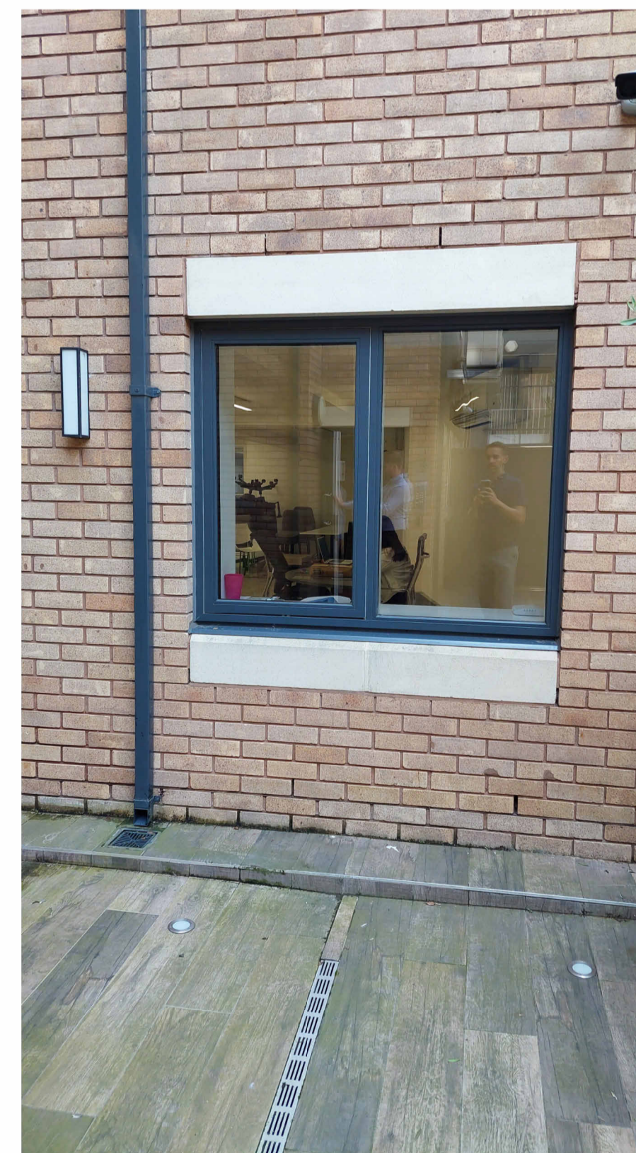
Existing patio photo showing current window WB.35 to be stripped out and converted into door DB.13
