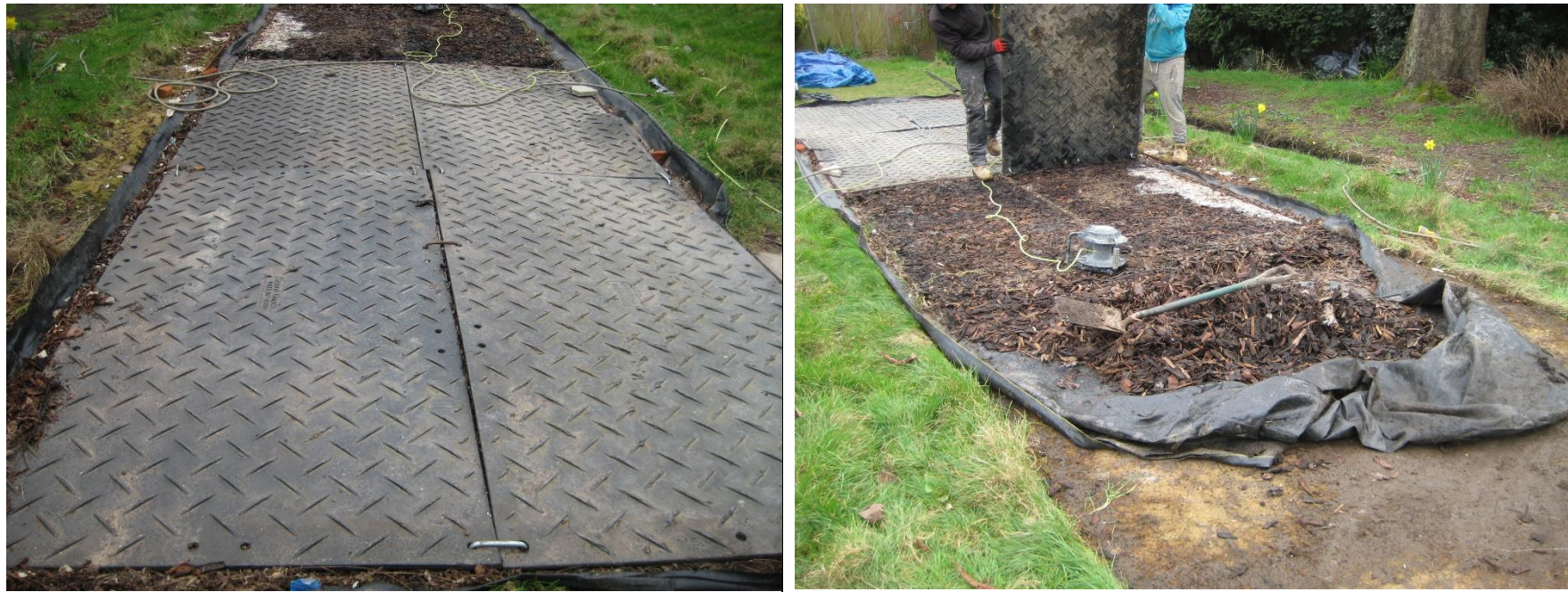
Fig 10 – Temporary ground protection is an effective way of allowing access through the RPA of retained trees. It must be installed prior to any on site activity and maintained for the duration of all works to be effective. Above left Tamla Trees project ground protection in place and above right being removed following the completion of site works. (Note: depending on the length of time it is in place it will adversely affect underlying grass ground cover which will need reseeded/ turfed accordingly)
