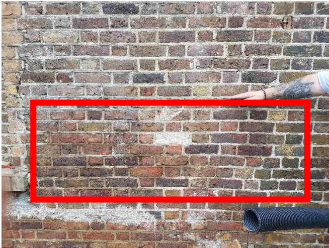
Brickwork to gable wall of Doughty Cottage after cleaning down. Note mix of yellow, red and dark bricks.
