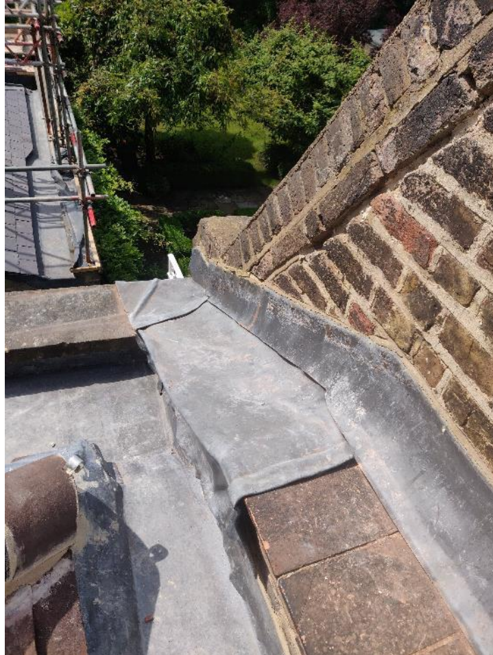
Flank wall to 51 – Awkward detail at south end which will require confirmation once parapet revision complete.
