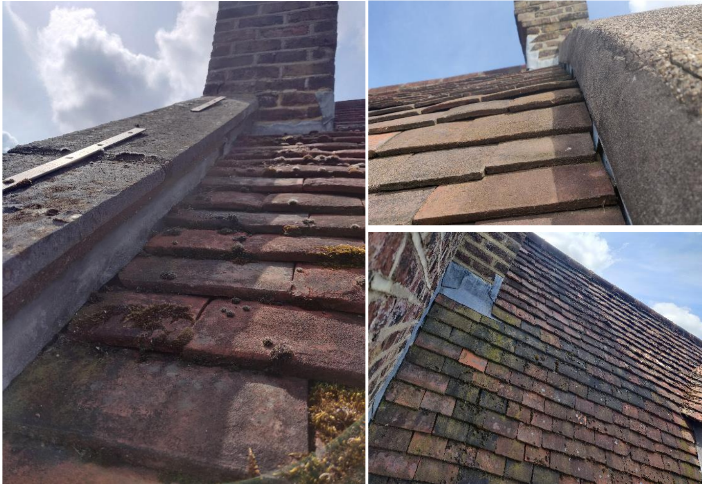
Left: Rear of parapet detail at detail A. Top right: Rear of parapet at Detail C. Bottom Right: Rear of parapet at Detail B.
