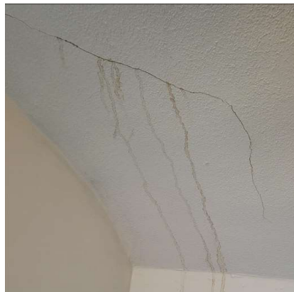
visible cracks and water marks
