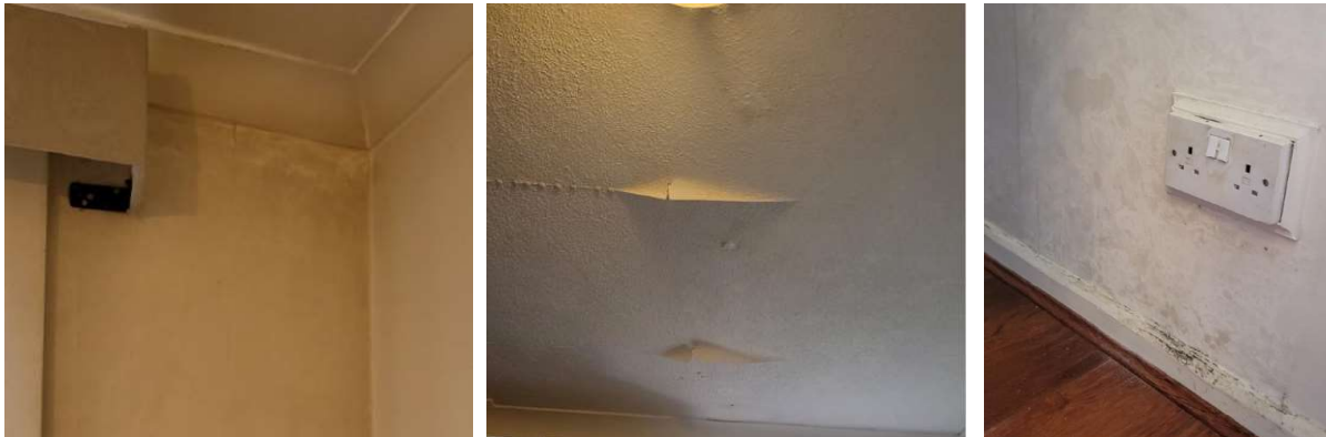
Ingress of water and damp on ceilings and walls
