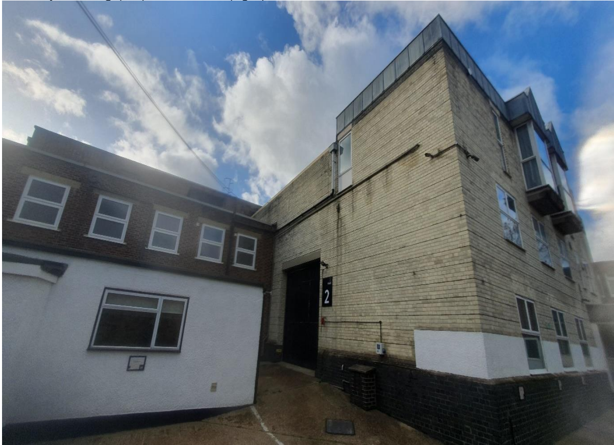
Plate 13: Image showing another part of the north-east elevation of Block C with one-storey ancillary building (left) and offices (right).
