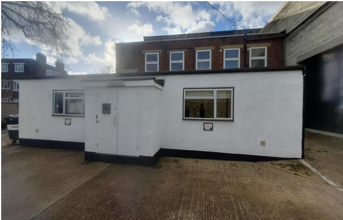
Plate 14: Image showing the north-east elevation of the one-storey ancillary building to be demolished within Block C .
