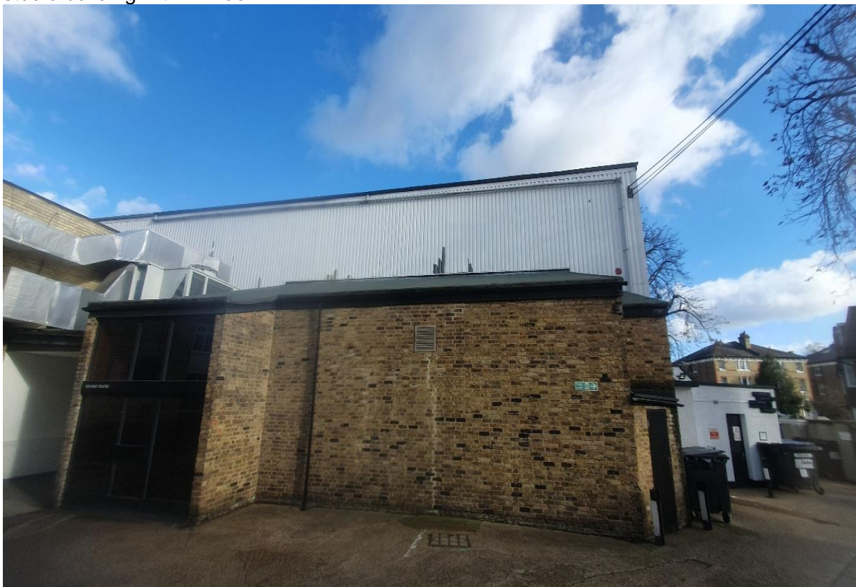
Plate 20: An image showing the south-east elevations of the one-storey lean-to and the studio building within Block F .
