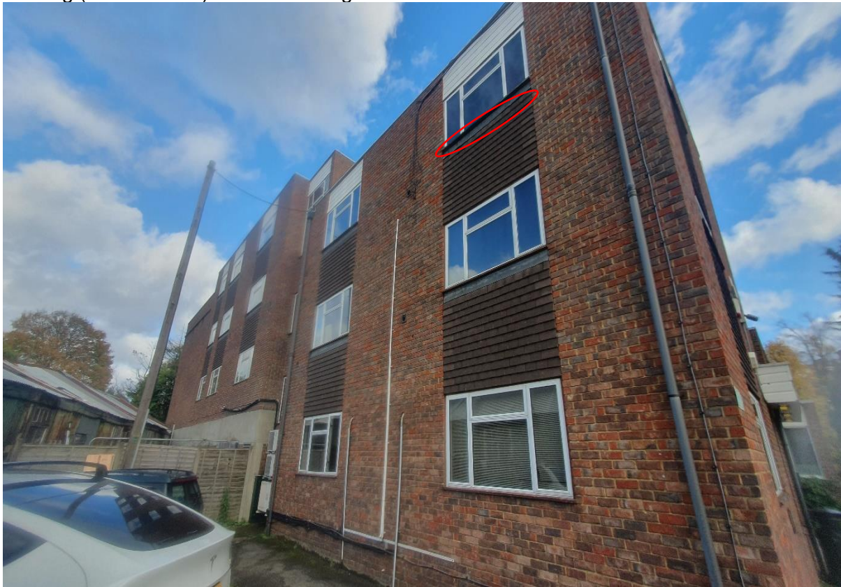
Plate 29: An image showing the north-west elevation of Block H with gaps under lead flashing (circled in red) above cladding.
