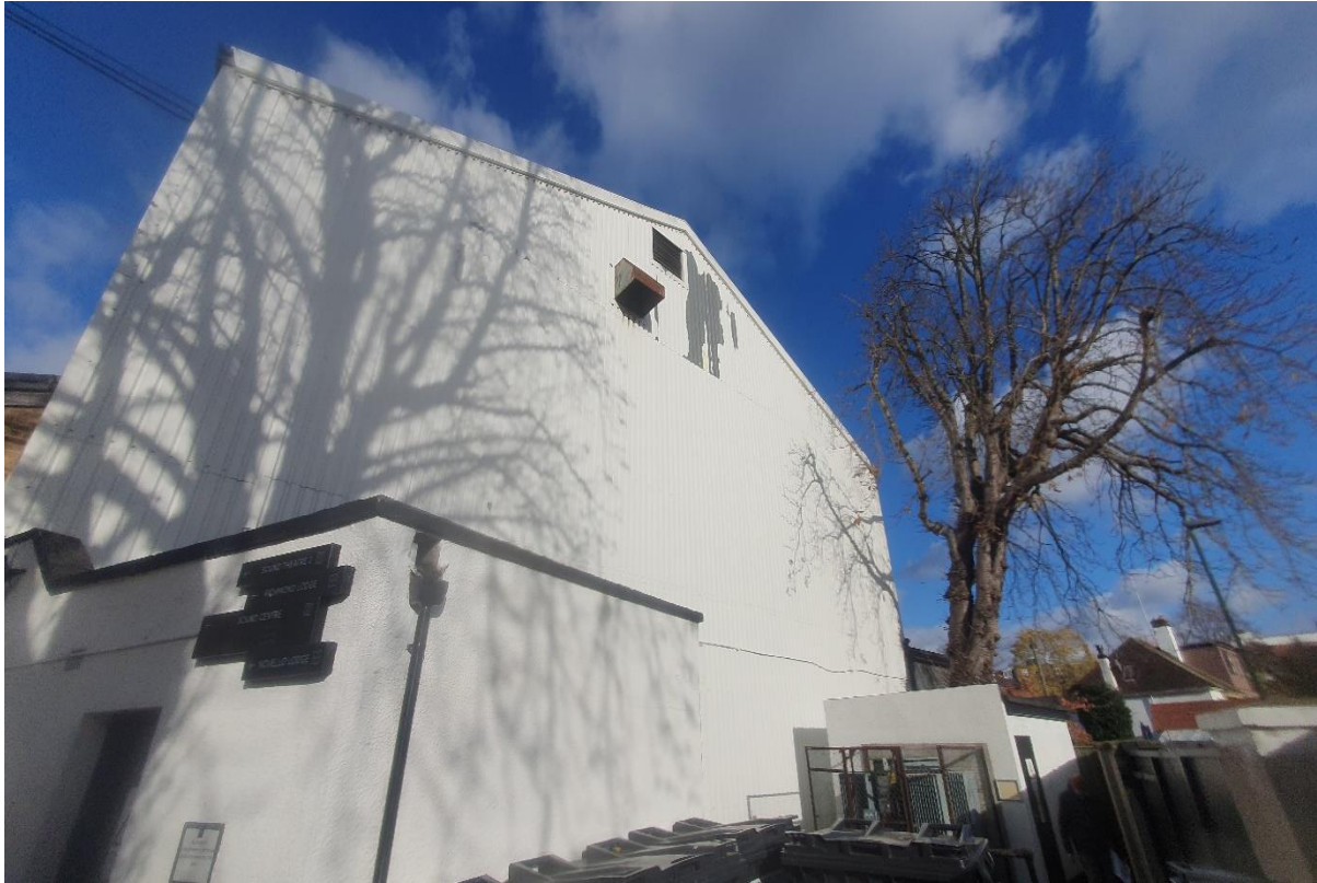
Plate 19: An image showing the south elevations of the studio building and one-storey units within Block F .
