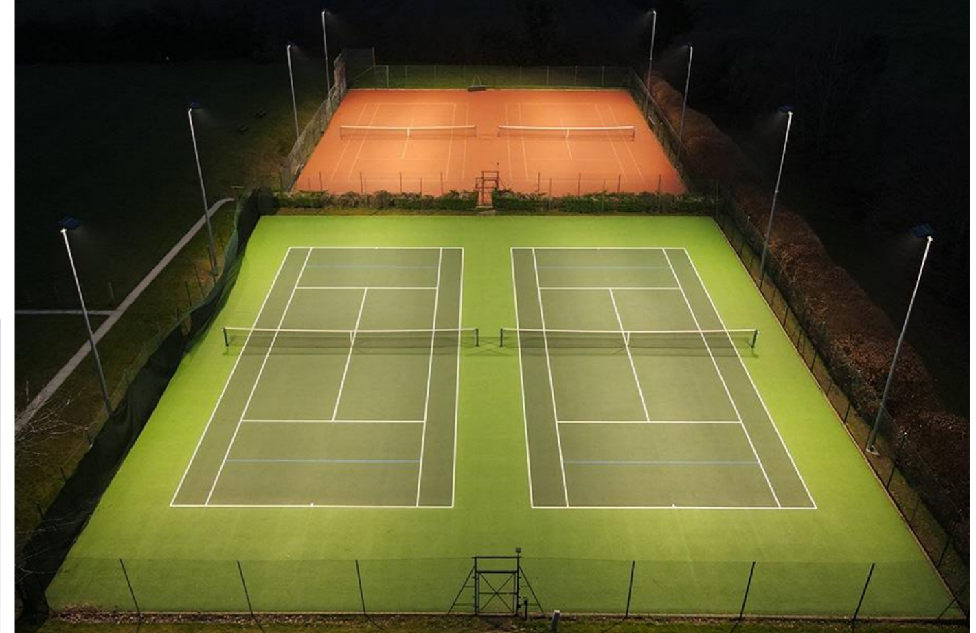
Column mounted floodlights – Illustrative Image.
