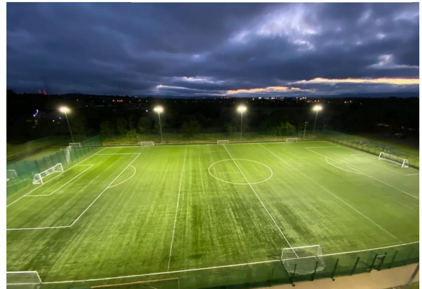
Column mounted floodlights – Illustrative Image.
